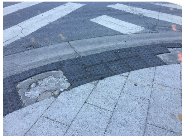
Figure 40: Example of a damaged detectable warning surface at the intersection of Fenton Street and Wayne Avenue.
