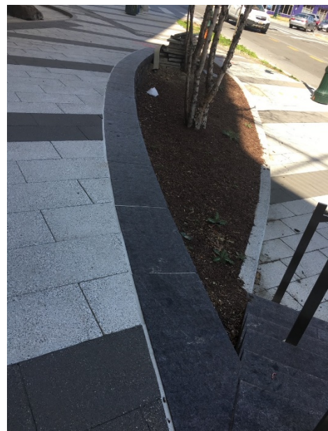
Figure 45: Unfenced wall drop off on the approach to the Fenton Street library entrance.
