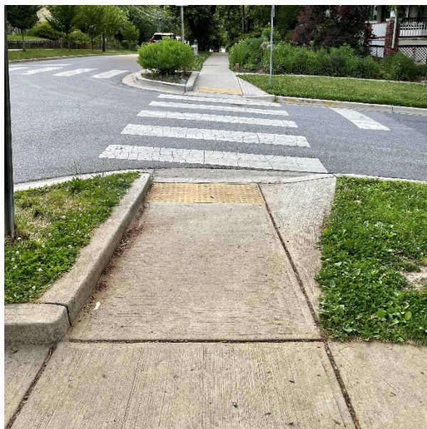
Figure 5: Example of a vertical curb incorporated into a curb ramp design in Takoma Park. This design includes multiple tactile cues for orientation and alignment, including: 1) a detectable change in slope indicating a transition from the sidewalk and roadway; 2) a detectable warning surface marking the end of the curb ramp; and 3) a vertical curb incorporated into the curb ramp design that can be used for pedestrian alignment with the crosswalk.
