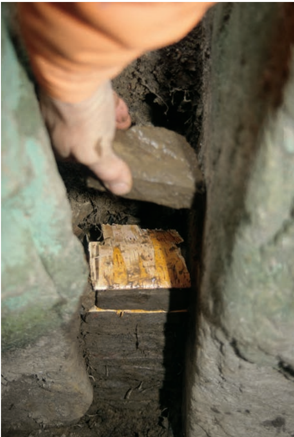
Fig. 1. An experiment with the rebuilding of dry-walling using fresh birch bark. The lower part of the dry-walling is original, while the upper two courses of sandstone flags are modern additions (photo: T. Dehn).
