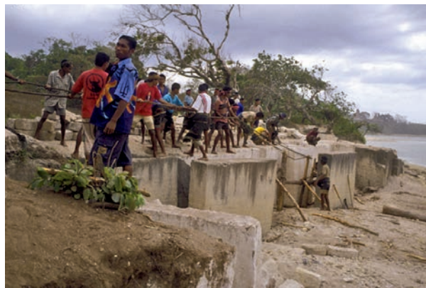
Fig. 6. Removing a limestone slab from a quarry in Kodi, West Sumba (photo: R. Adams).
