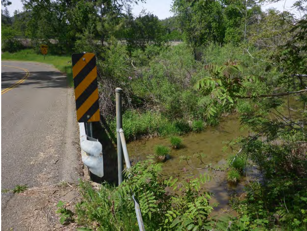
West Fork Stillwater Creek at Old Oregon Trail North, view to west. April 15, 2020.
