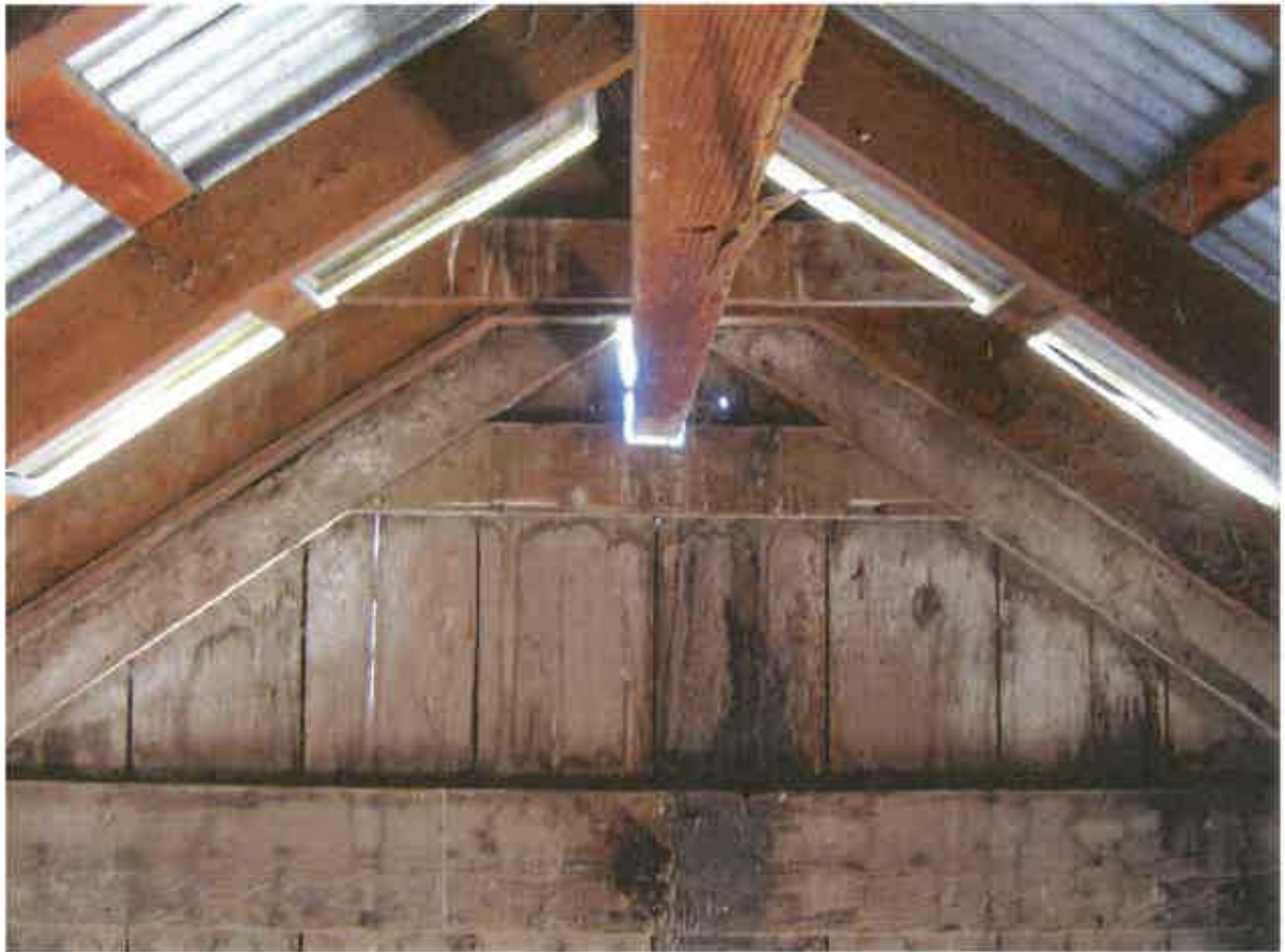
Figure 52. Watermarks found throughout the interior face of the wood siding.
