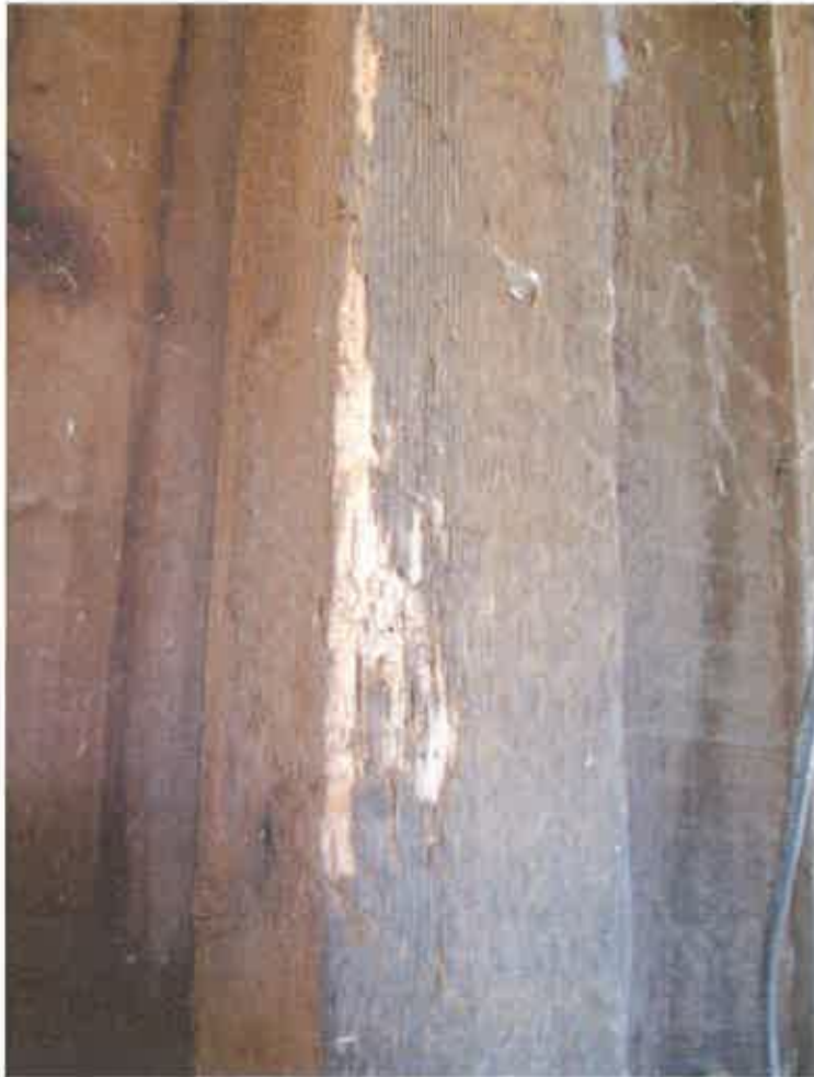
Figure 53. Typical surface deterioration from insect infestation at the timber posts.
