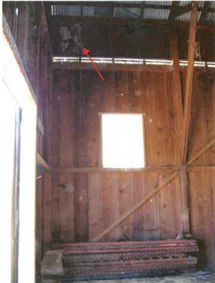
Figure 64. Water stains on the wood boards at the northeast corner of the center aisle. And old rail track stored on the fragile floorboards in the center aisle.
