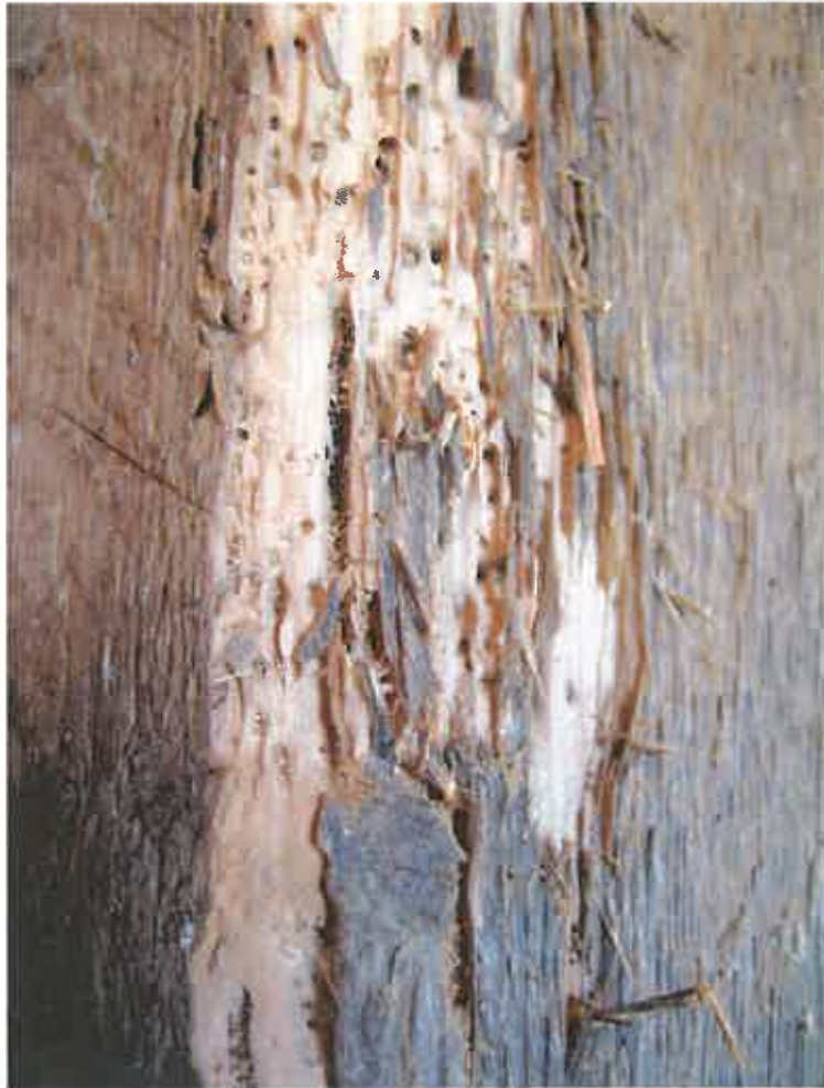
Figure 54. Detail view of the surface deterioration caused by insect infestation.
