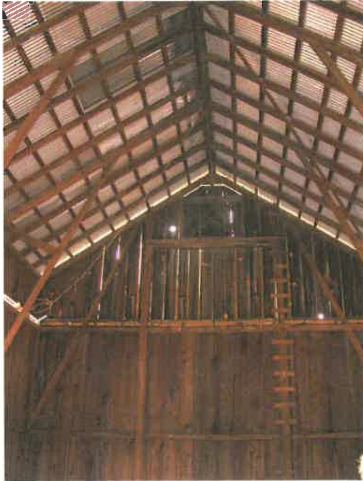
Figure 24. Interior view of the south wall and roof framing from the center aisle.
