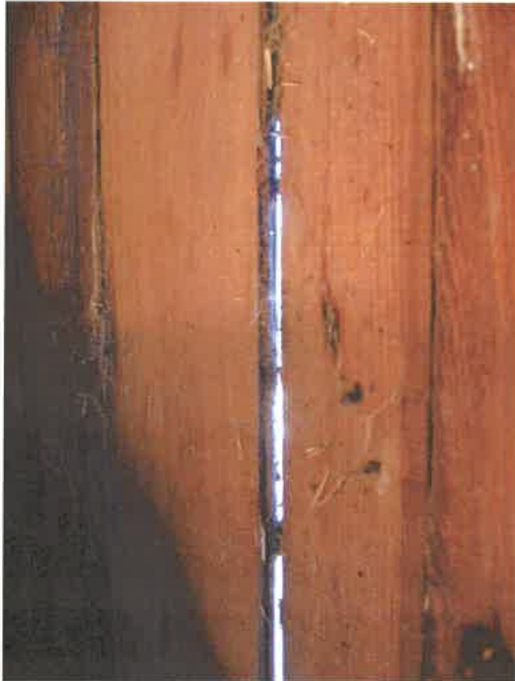
Figure 51. Typical gap between exterior siding.
