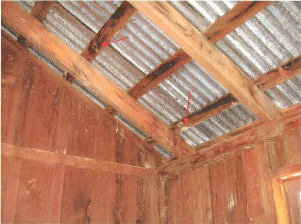
Figure 65. Deterioration of the roof framing system at the rear storage areas.
