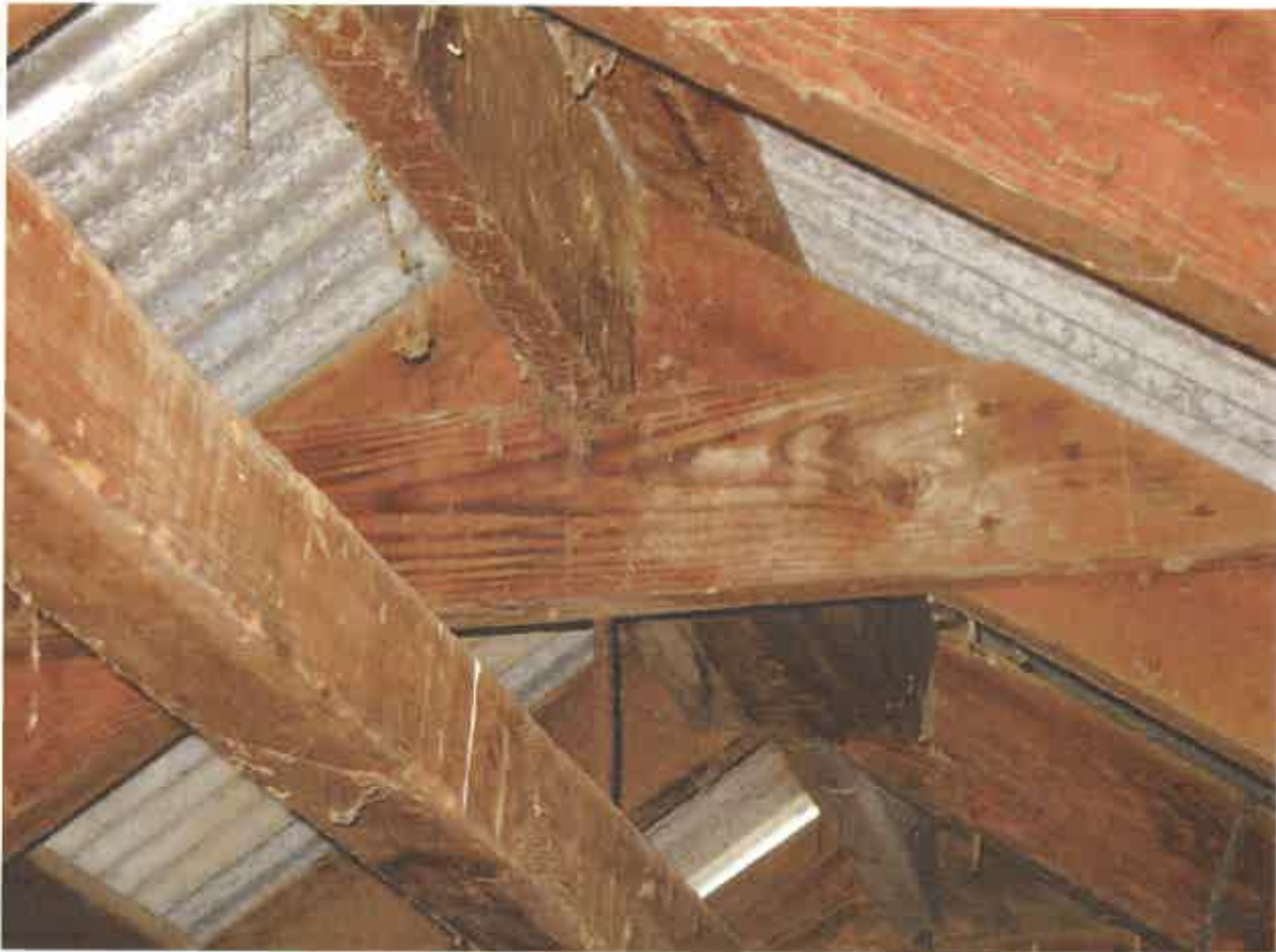
Figure 27. Roof framing system at the center aisle showing where rafters join the ridge beam. Square member below used as a track for the hoist.
