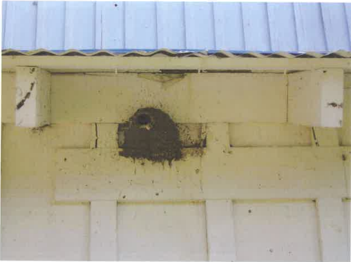
Figure 49. Bird nest found near the roof framing system at the exterior south elevation .
