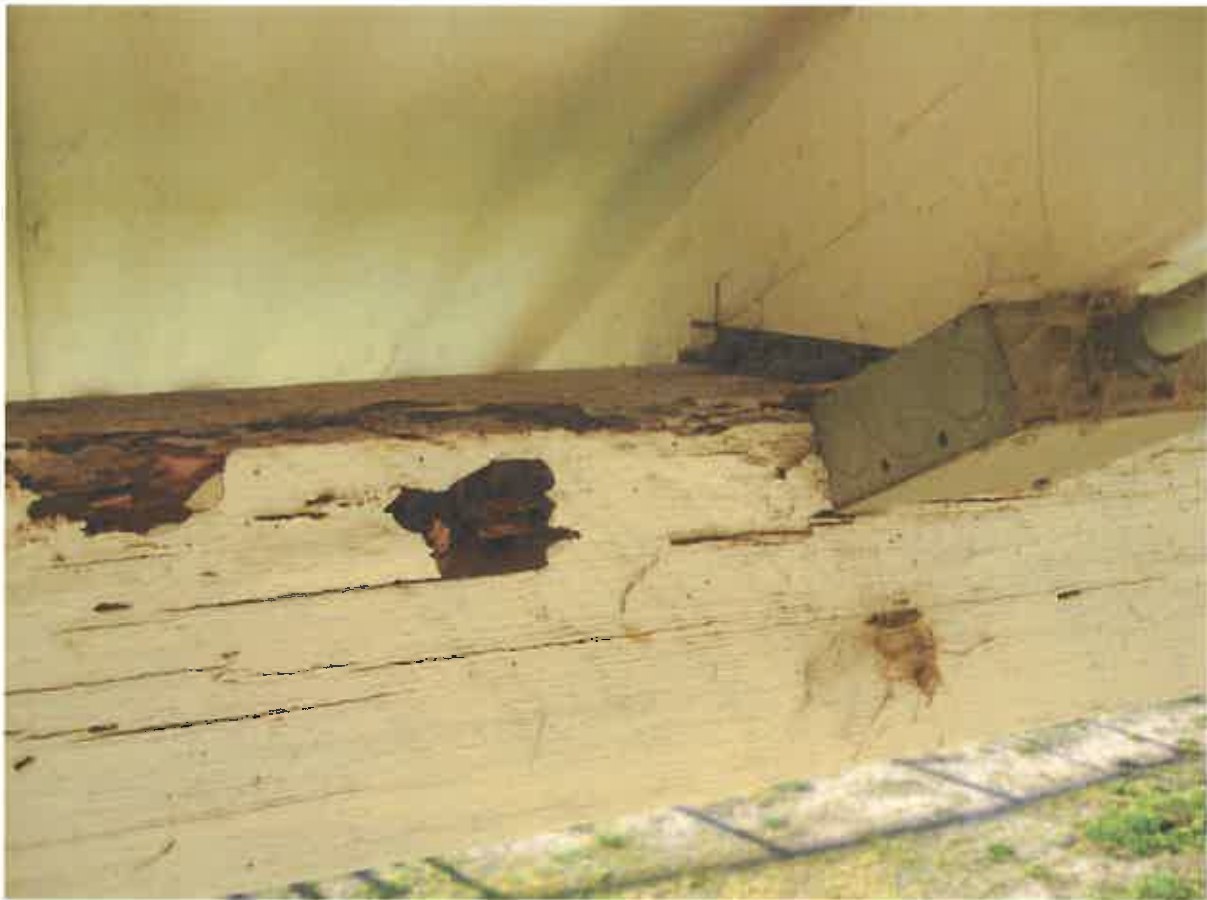
Figure 61. Deterioration of roof framing system at the east aisle caused by pests.
