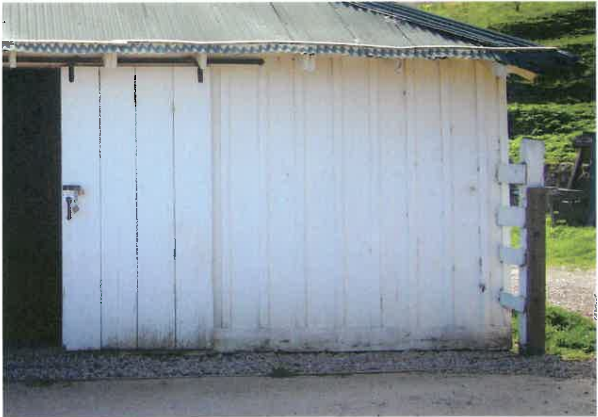
Figure 46. Soiling at the base of the exterior siding.
