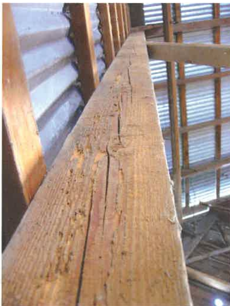
Figure 55. Splits found on timber posts.
