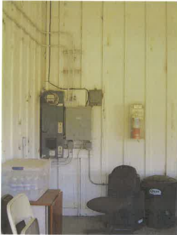
Figure 35. Main electrical panel located on the west elevation wall of the east aisle.
