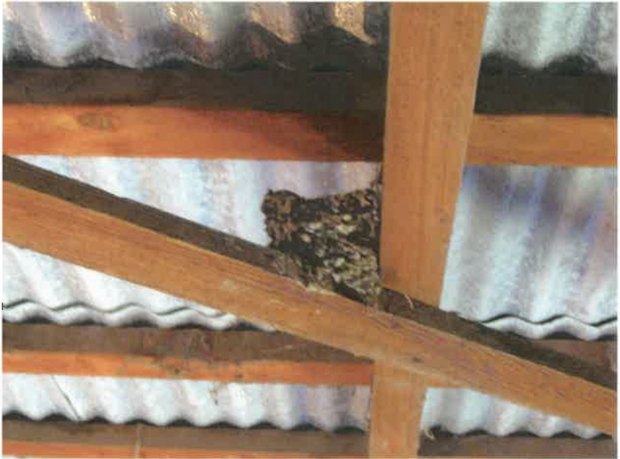
Figure 62. Bird nest found nestled within roof framing system at the center aisle.
