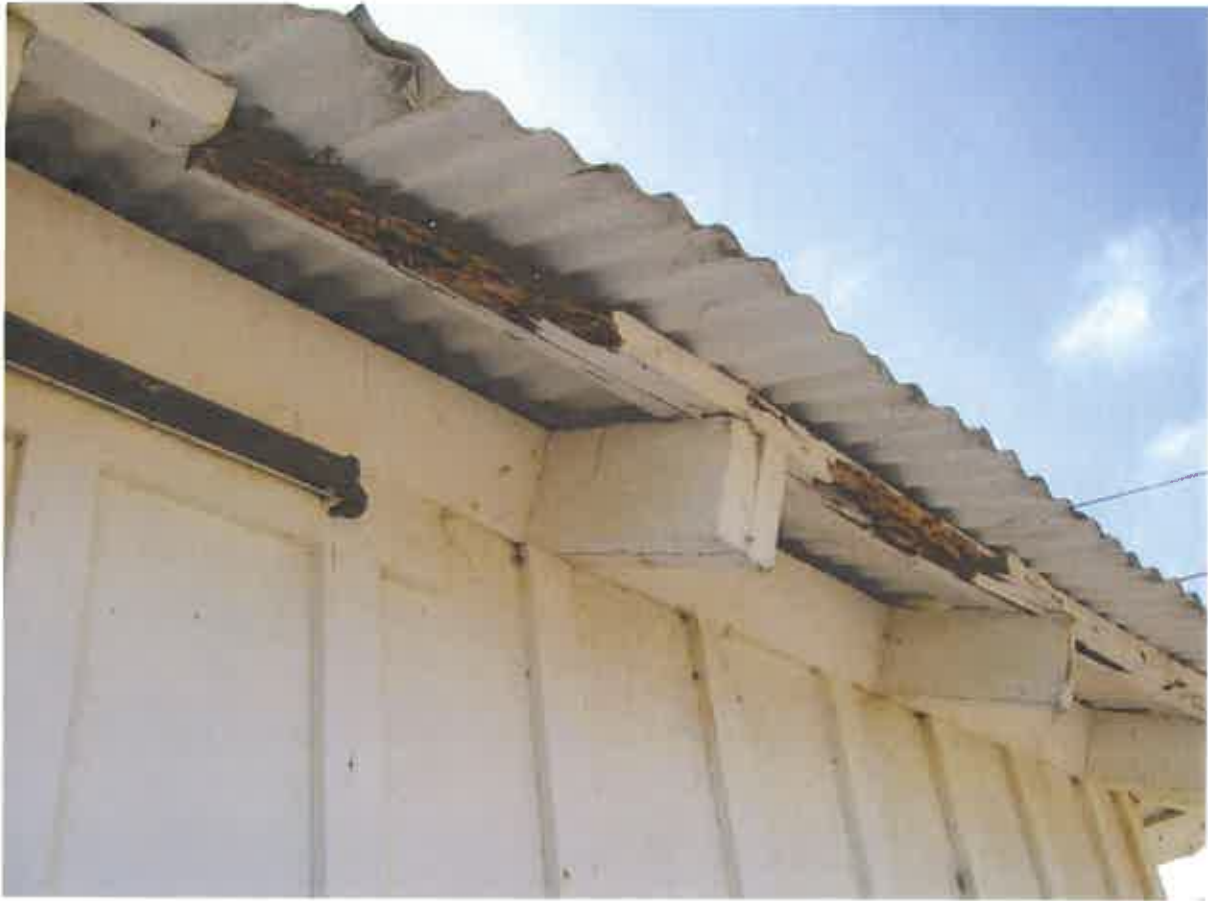
Figure 59. Deterioration of sleepers at roof framing system.
