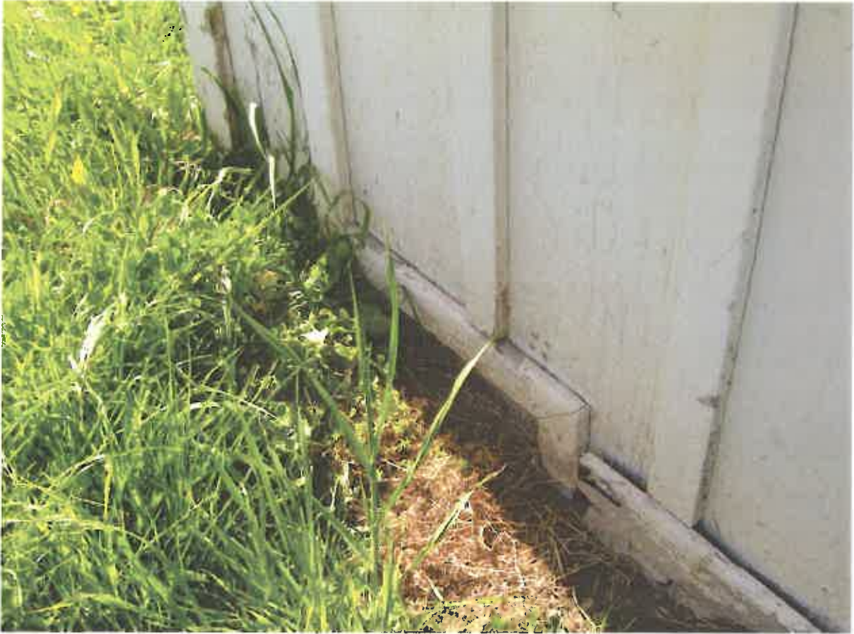
Figure 47. Soiling at the base of the wood siding.
