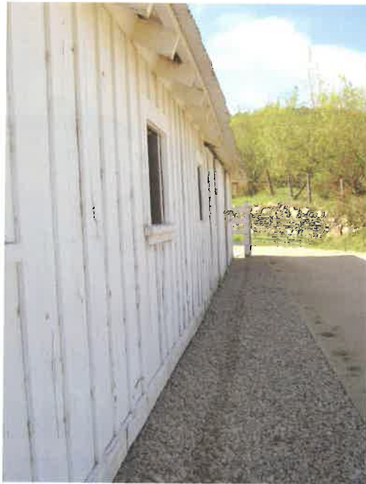
Figure 9. French Drain at the west elevation.
