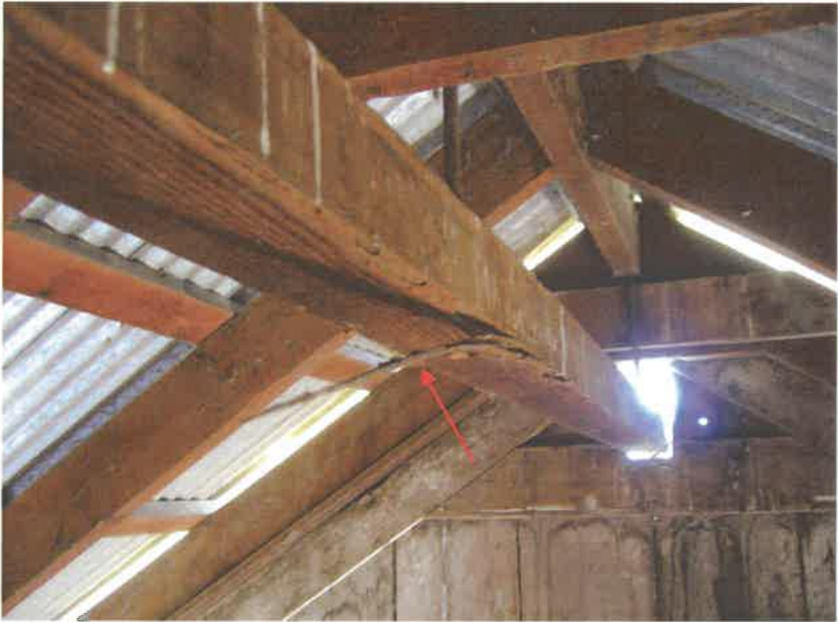
Figure 57. Surface deterioration showing separation of wood fibers at the hoist rail used to move the hay fork.
