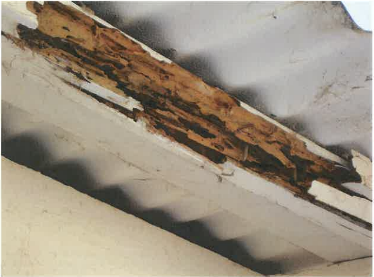
Figure 60. Detail view of deterioration at sleepers.
