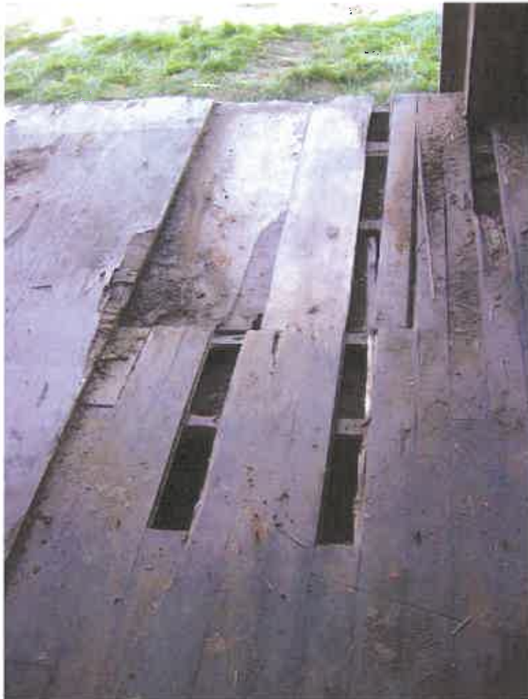
Figure 63. Deteriorated floorboards at the center aisle.
