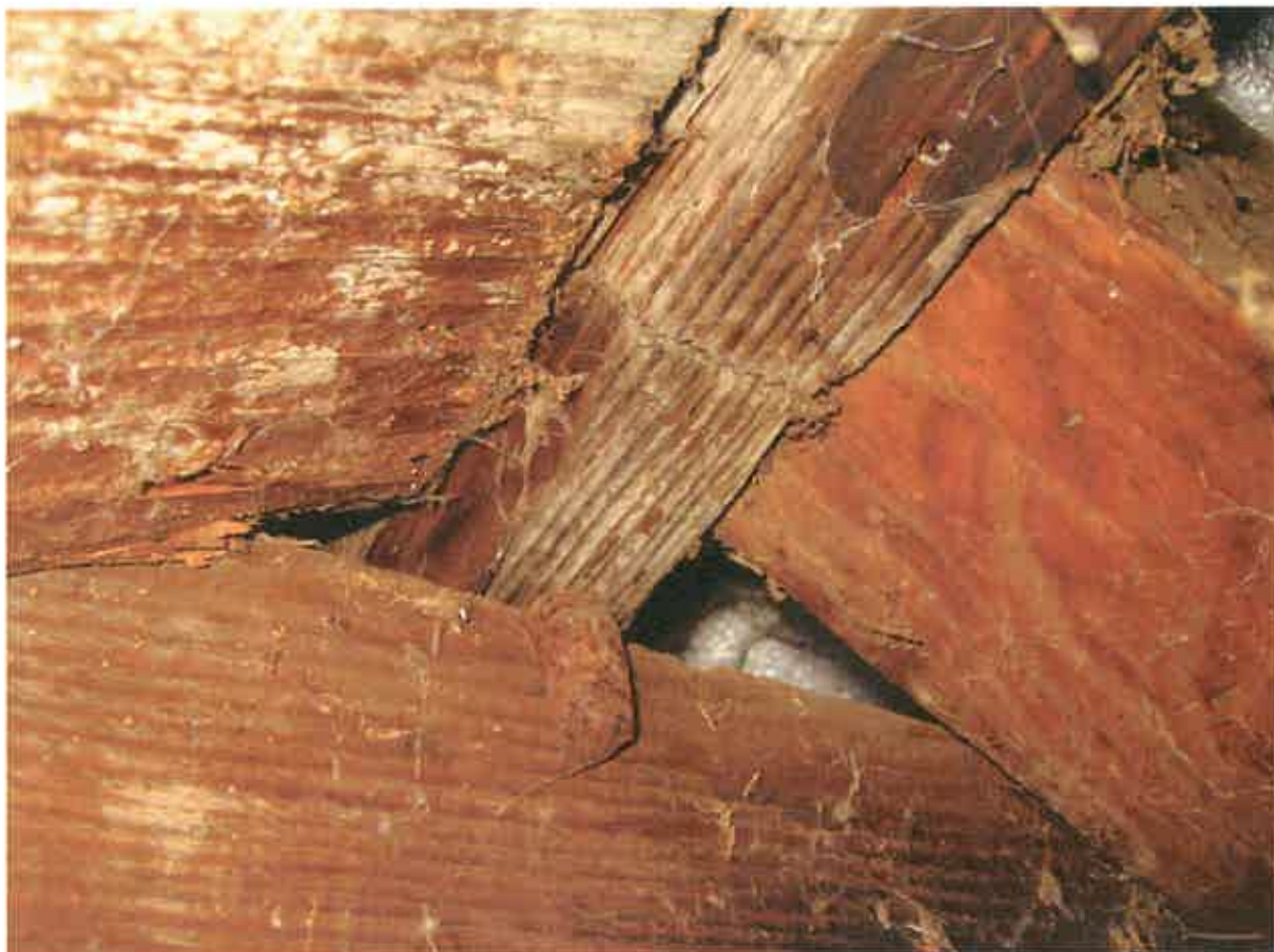
Figure 56. Deterioration at the roof framing system.
