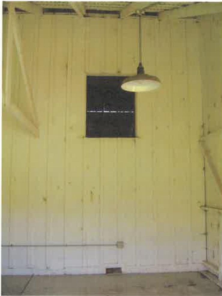
Figure 33. Opening at the east elevation wall in the east aisle looking into the center aisle.
