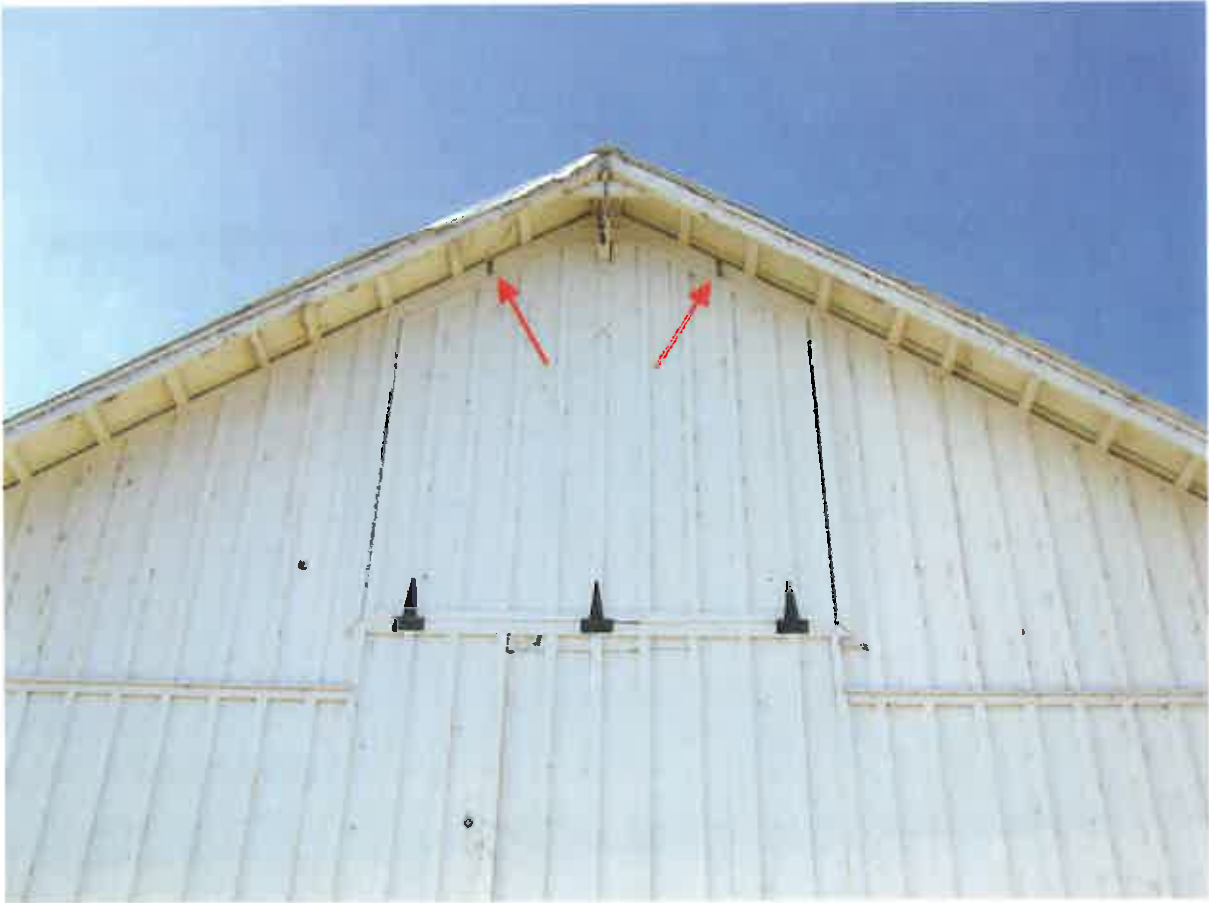
Figure 12. Hay loft door located below the gable roof at the north elevation.
