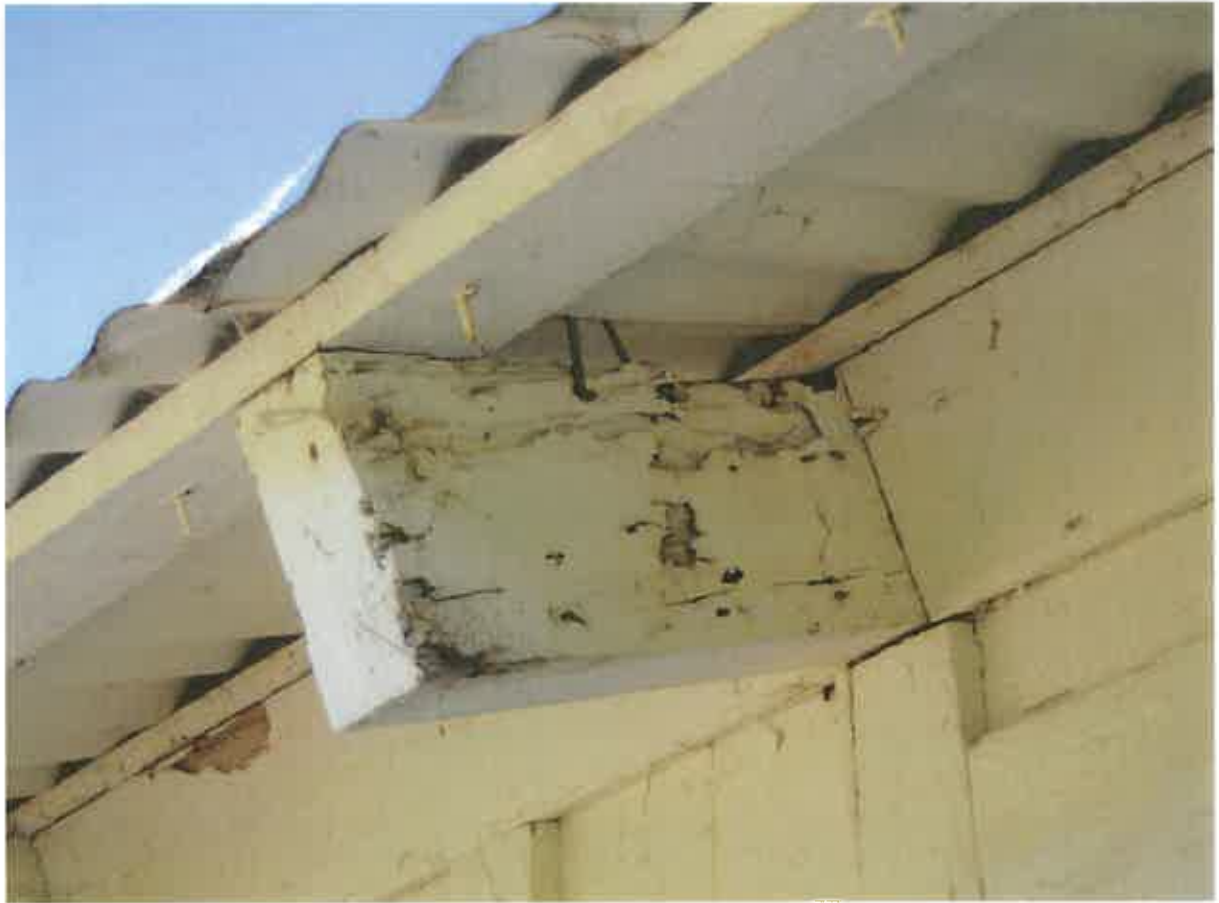
Figure 58. Typical deterioration of roof rafter ends.
