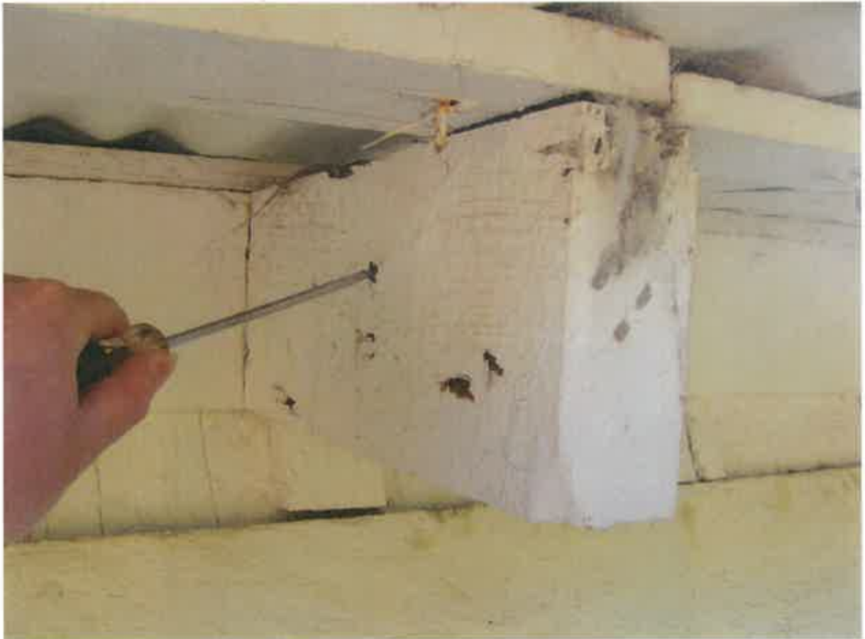
Figure 42. Testing by probes conducted during the field investigation. View of a rafter exposed to the exterior.
