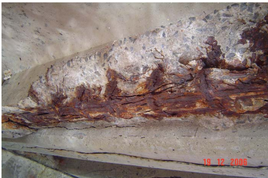
Figure 17: Typical cracking and deterioration under U beams
