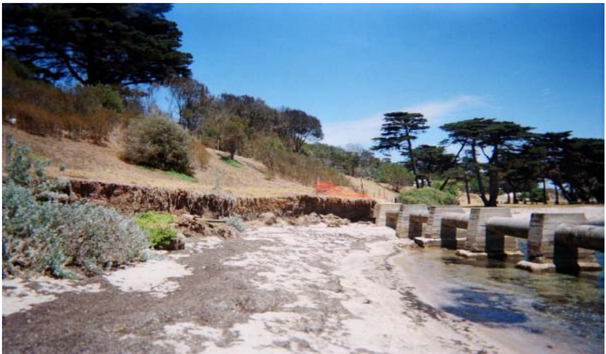
Figure 5 Significant scour near stormwater outfall.
