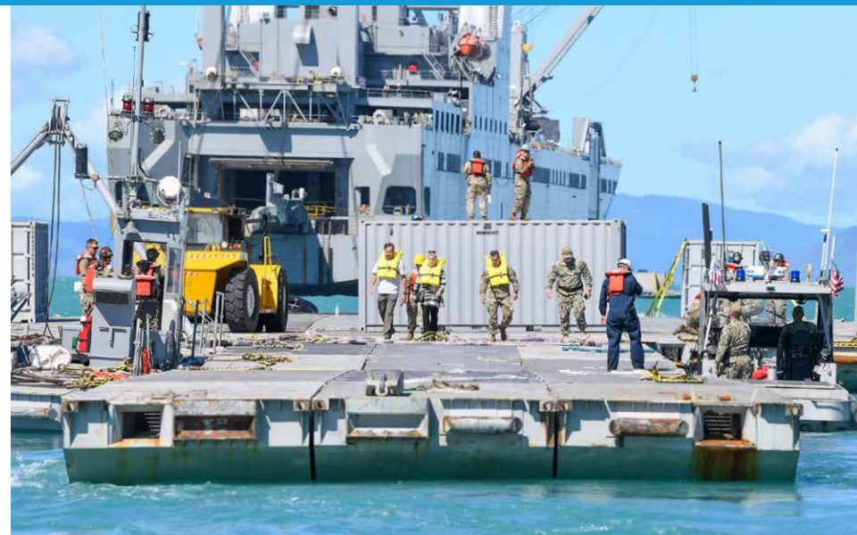
Secretary of the Army, Hon. Christine Wormuth, visits Army mariners assigned to the 368th Seaport Operations Company and 331st Transportation Company construct a causeway adjacent to the MV Maj. Bernard F. Fisher off the coast of Bowen, Australia. (U.S. Army photo by Sgt. David Resnick)
