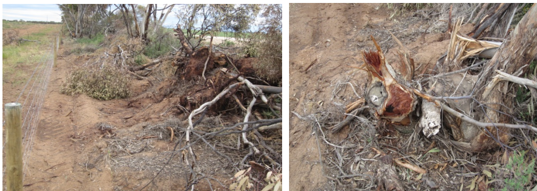
Figure 26: Poor relocation of a fence line
