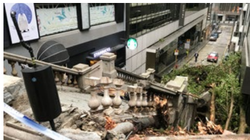
6 古蹟因大樹倒塌受到嚴重損毀 The Monument was seriously damaged by the collapse of a large tree.
