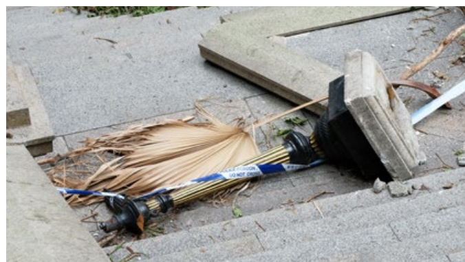
8 折斷的鑄鐵煤氣路燈燈柱 The broken cast-iron column of a gas lamp
