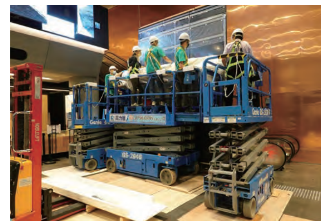
11 工作人員操作剪刀式升降工作平台及堆高車的實況。 Actual setup with the mentioned lifting equipment and manpower deployed during operation.
