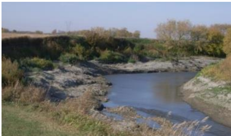
Bank failure along a Red River Basin stream
