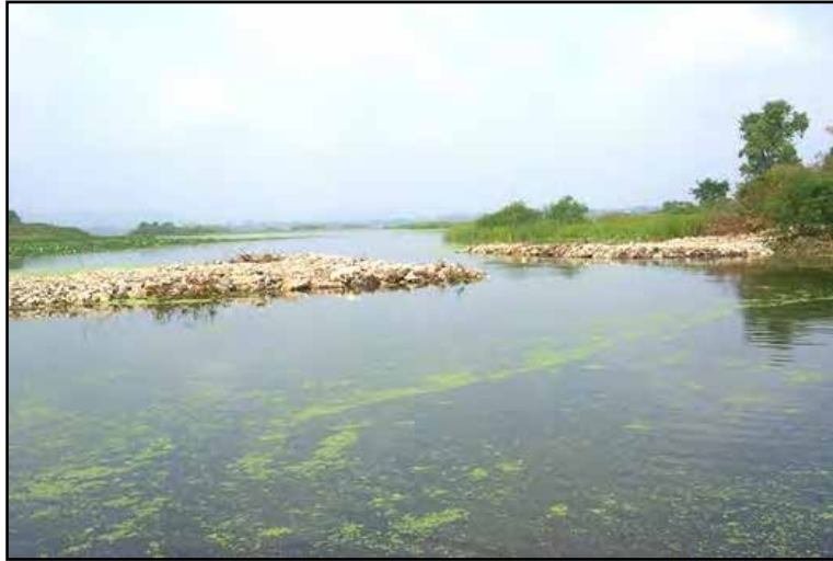
Photograph 7-1. Partial Closure Structure at the Weaver Bottoms Secondary Channel, Pool 5 (Jon Hendrickson, MVP 2005)
