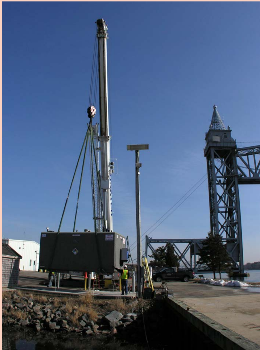
Crane moves new tank system into place at the Cape Cod Canal.
