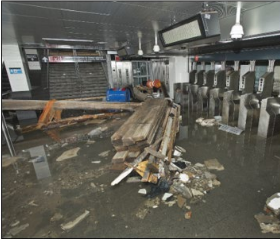
MTA New York City Transit South Ferry subway station after it was flooded by seawater during (Cashin, 30 Oct 2012)
