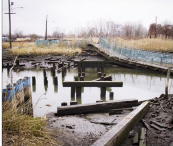
Destroyed popular pedestrian bridge at Liberty State Park, NJ (Arias, 23 Sep 2013)
