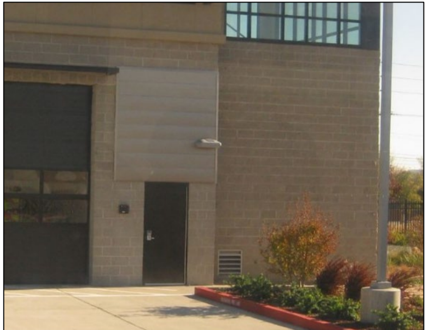
Figure 34: Wet floodproofing in Sacramento, CA.
