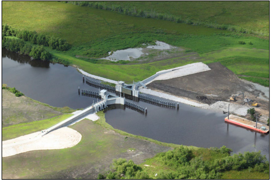
Figure 30: Tide gate along a navigable waterway in Louisiana.
