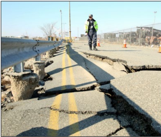
Damage to main roadways used for connecting the Ports moving commerce in Newark, NJ (DuBrowa, 12 Dec 2012)
