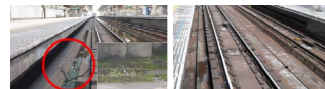
Removal of moss from tracks using high-pressure washers at Tengachaya Station (before washing on left, after washing on right)
