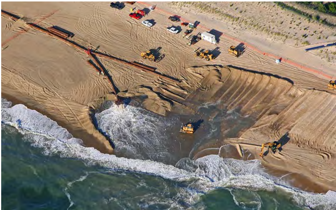
Figure 3-3. A Typical Beachfill Operation along the Delaware Atlantic Coast. (Source: Great Lakes Dredge and Dock Company website accessed at: http://www.gldd.com/company/projects/coastal-protection/ on 5/7/2015)
