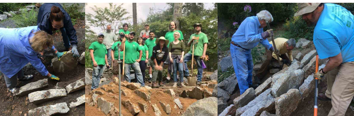
An army of volunteers including those from the gardens (left), Citrix Coporation (center) and Master Gardeners (right) constructed the garden in record time.
