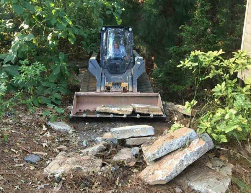
The first delivery of what used to be the sidewalk around City Hall in Kennesaw, Georgia. Eventually, 14 tons of trash concrete were delivered and installed.
