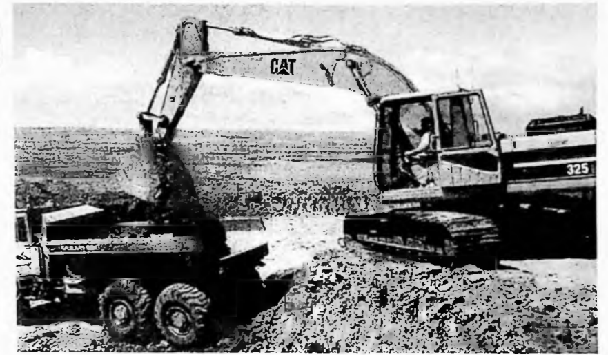
Above: raw material is loaded into dumper trucks 500 metres from the end of the road.
