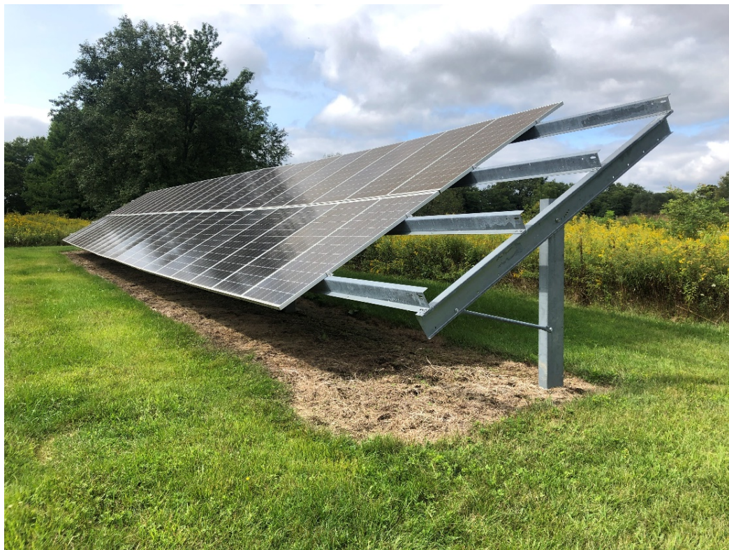
A solar array that has native plants surrounding the site but is mowed around and sprayed underneath the panels to prevent vegetation. If the solar arrays were higher off the ground, a native seed mix with a growing height of no more than 36 inches can be planted underneath. © Kim Steinberger/TNC
