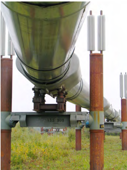
More than half of the Alaska pipeline is elevated above ground to allow wildlife passage beneath, and to prevent permafrost thawing. The pipe supports in some sections are refrigerated to prevent conduction of heat into the ground. Photo by Derek Ramsey.
