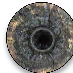
Erosion in chamber
