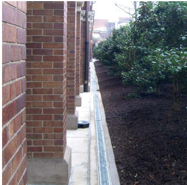
Trench drains along the Building arcade help to control stormwater runoff at the Main Post.
