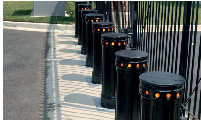
Removable bollards provide flexibility for intermittent uses such as access points.
