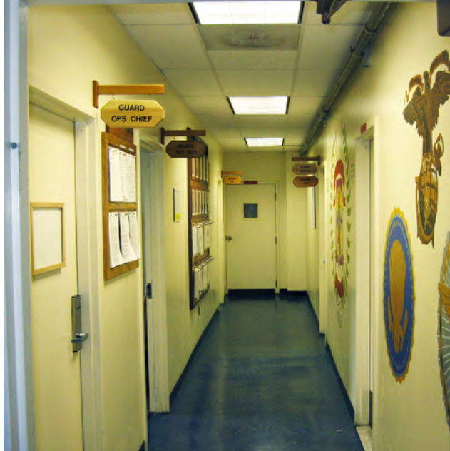
Years of modifications to Building 8 have led to compartmentalized, isolated, and inflexible use of the space.
