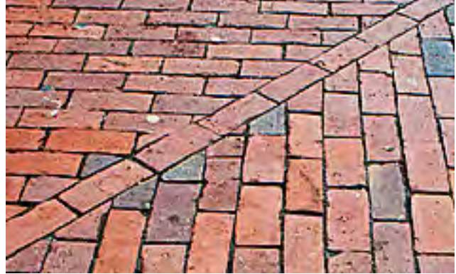
Context-sensitive solutions include appropriate size placement and material selection to integrate with surrounding historic streetscape of the Capitol Hill neighborhood.
