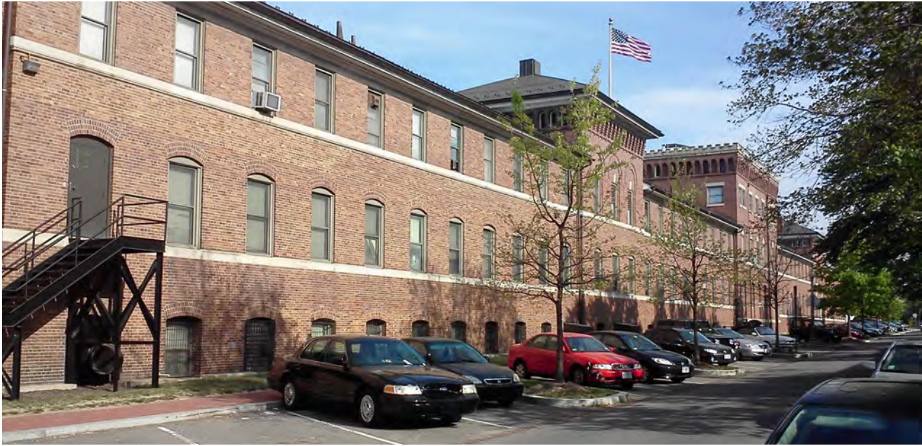
Non-compliant parking along 9th Street is within 17 feet of Building 8 and lacks a controlled perimeter.
