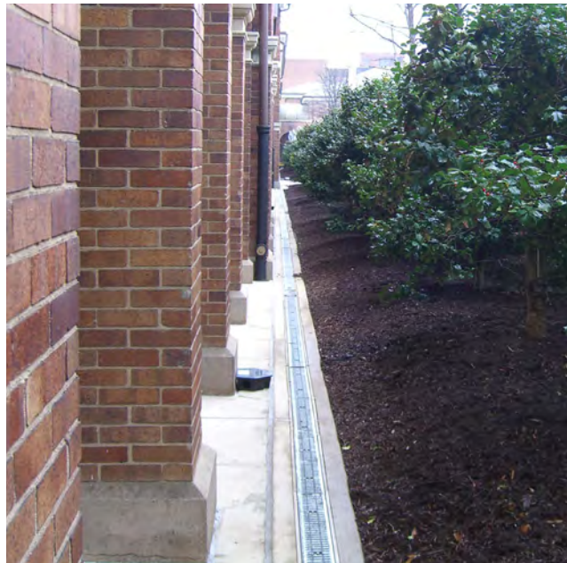
Trench drains along the Building arcade help to control stormwater runoff at the Main Post.
