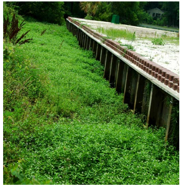
Alligatorweed clogging a drainage canal. (©Bridget Lassiter)
