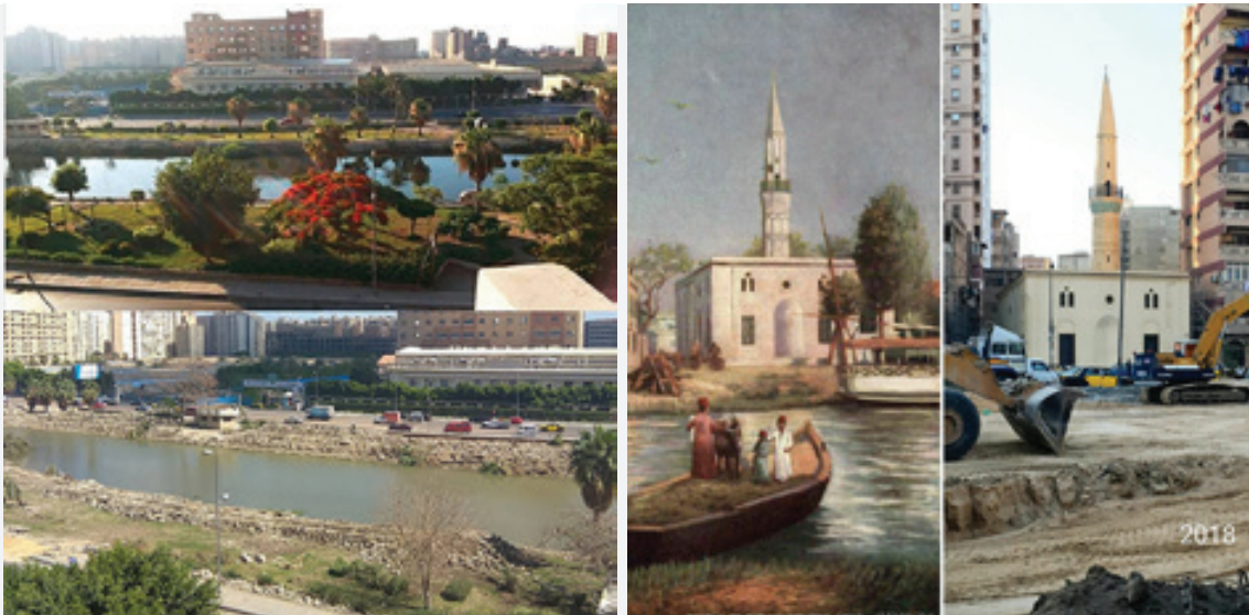
Figure 14: left: Before and after for new mahmoudia canal highway progress Right: demolishing the collective memory of "Ingi Hanim Mosque on Mahmoudia canal. Source: By researchers.
