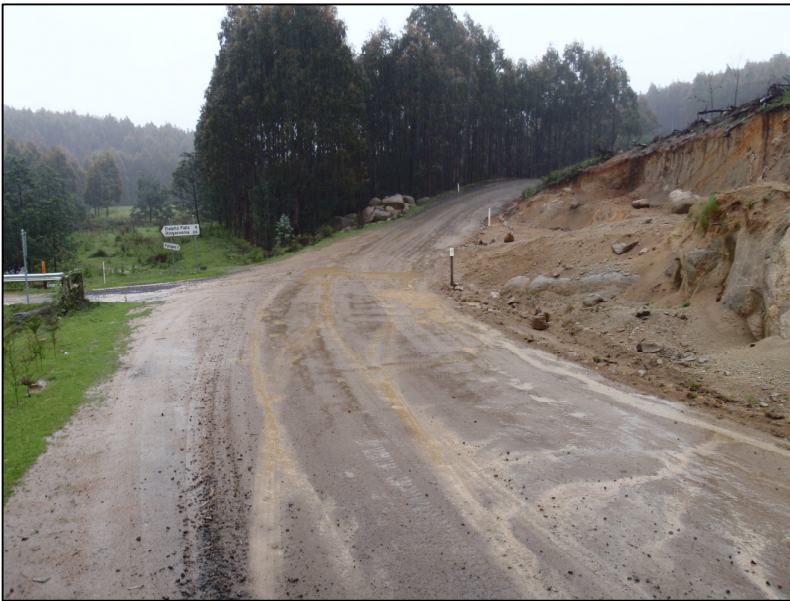
Figure 11 Turn off to Ralph Falls over South George River. Roadside erosion, the result of the bank being too steeply cut away. During heavy rain events wash of sediment into the river is inevitable. Bank could be battered more gradually and planted with low growing native grasses to stabilise it and reduce sediment loss and still allow sunlight to reach the road.
