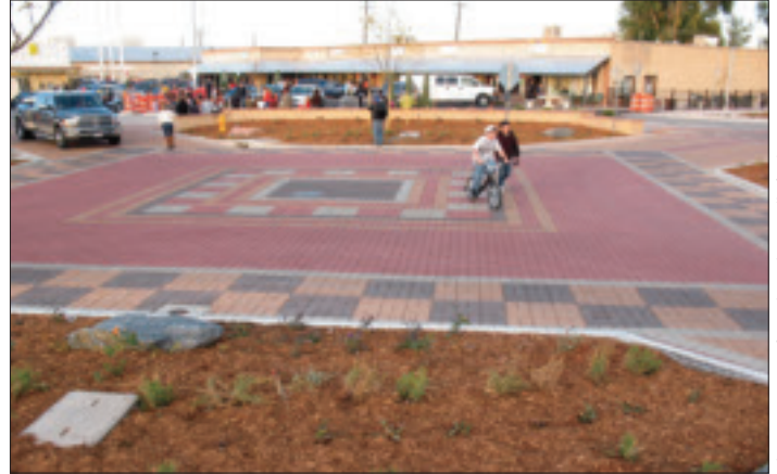
72nd Place and Monaco Street, after installation of the Derby Diamond intersection in 2011. Colored and textured pavement and curb extensions with landscaping slow traffic and make the intersection pedestrian-friendly.
