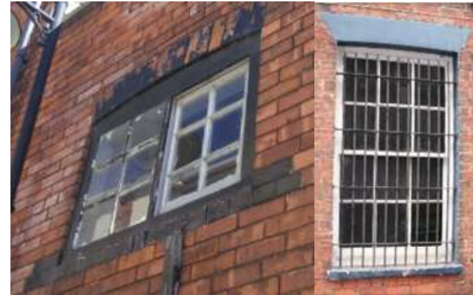
Left) 6/6 Yorkshire sliding sash on Wardall Street. (Right) Vertical box sash 6/6 on New Road.
