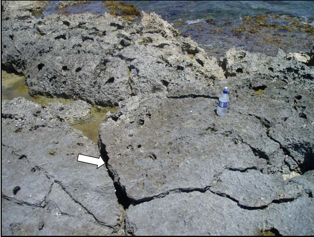
Plate 4 Joints associated with the White Bay Fault, exposed in the Falmouth Formation platform
