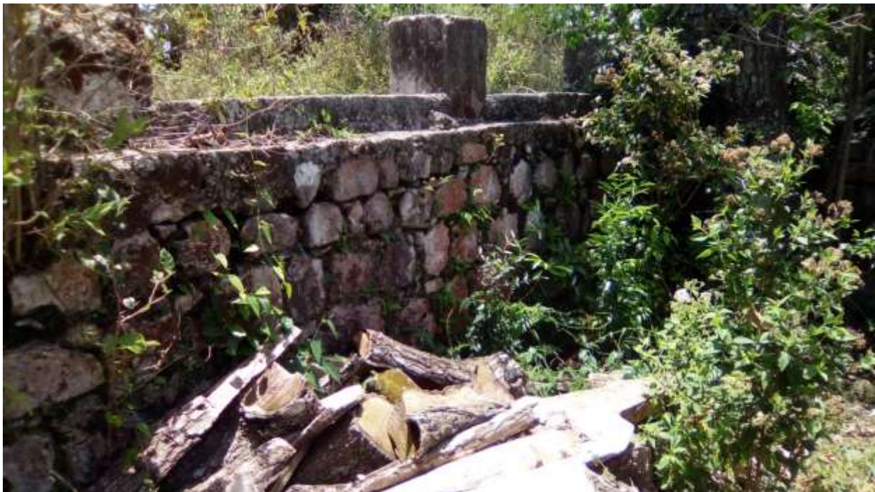
Figure 5-92: Part of the remaining wall and foundation of the Mitcham Greathouse
