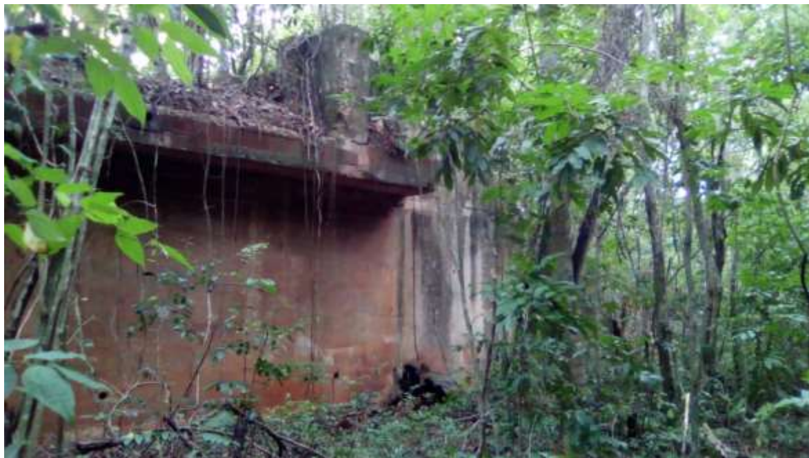
Figure 5-109: Remains of a retaining wall built along the railway in Fellowship
