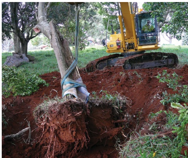
Figure 6.5 Transplanting Floydia praealta (Ball Nut) using the direct transplant method during construction of the Ballina Bypass. Monotypic genus is endemic to lowland subtropical rainforest between Nambour (Qld) and Ballina (NSW). (Photo: A Benwell)
