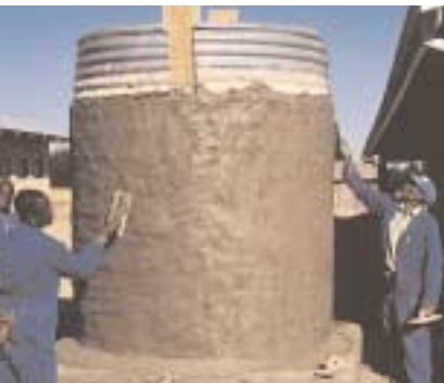
Village water tank in South Africa community development.
