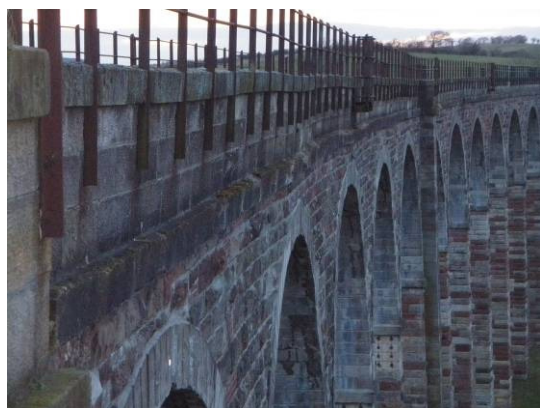
Figure 4.5: Mis-aligned stringcourse, Burnton Viaduct
