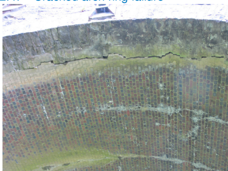
Figure 2.4: Cracked arch ring failure
