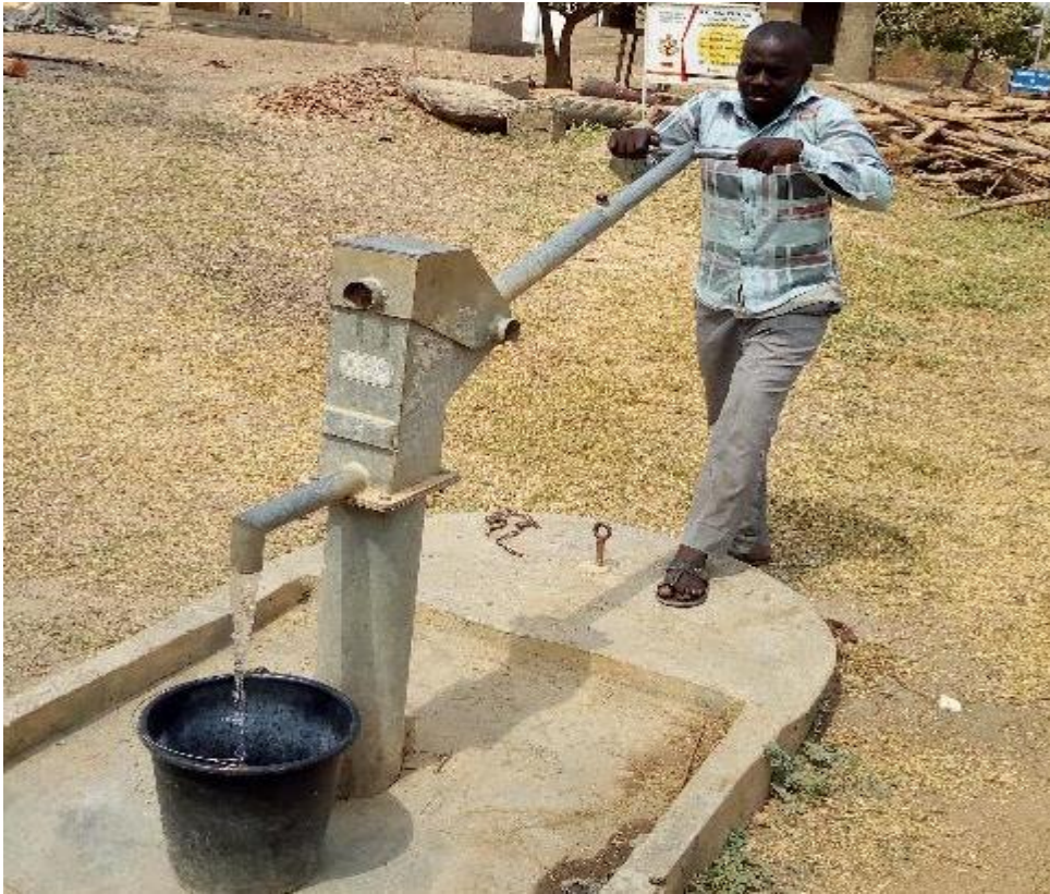
Plate 4.15: Manual borehole used in Ajaokuta community
