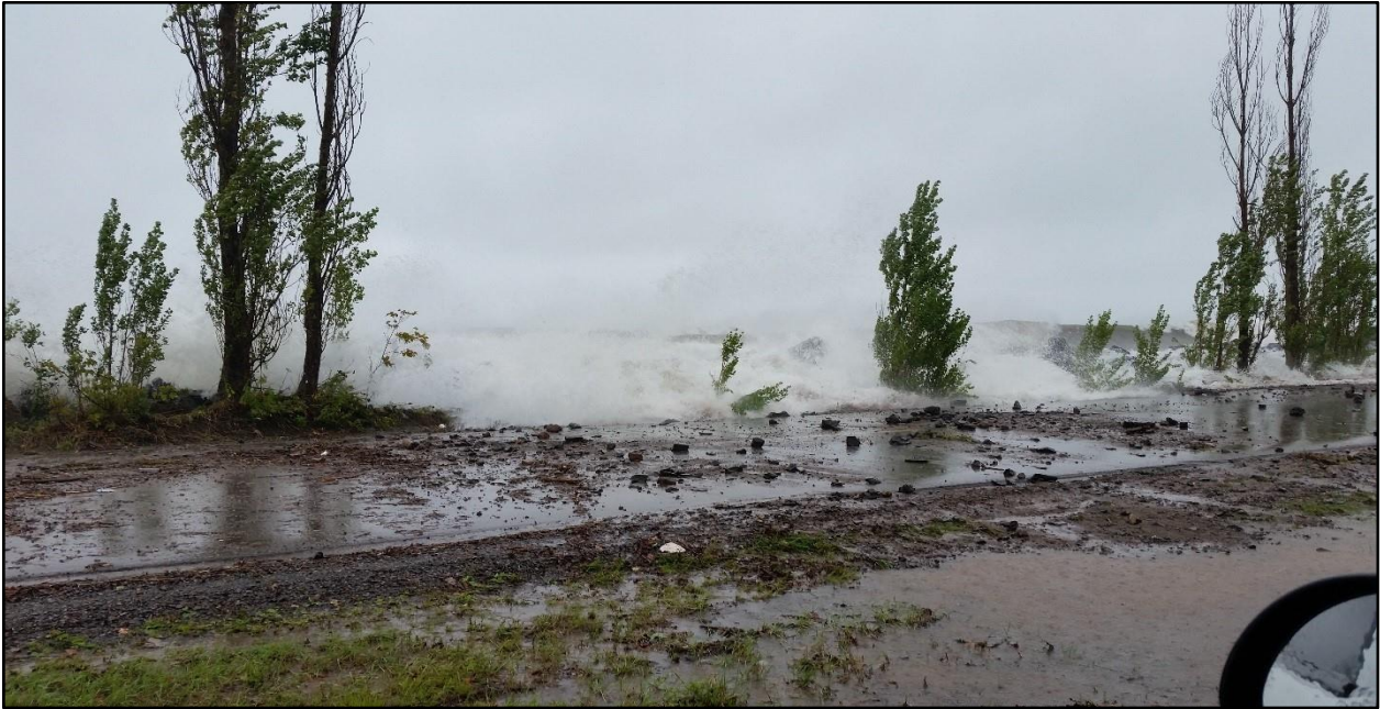
Figure 22. Lake Shore Boulevard during a large storm event. Waves are seen overtopping the existing revetment, scattering debris over the road. Image credit: Geraldine Grant, Superior Watershed Partnership.
