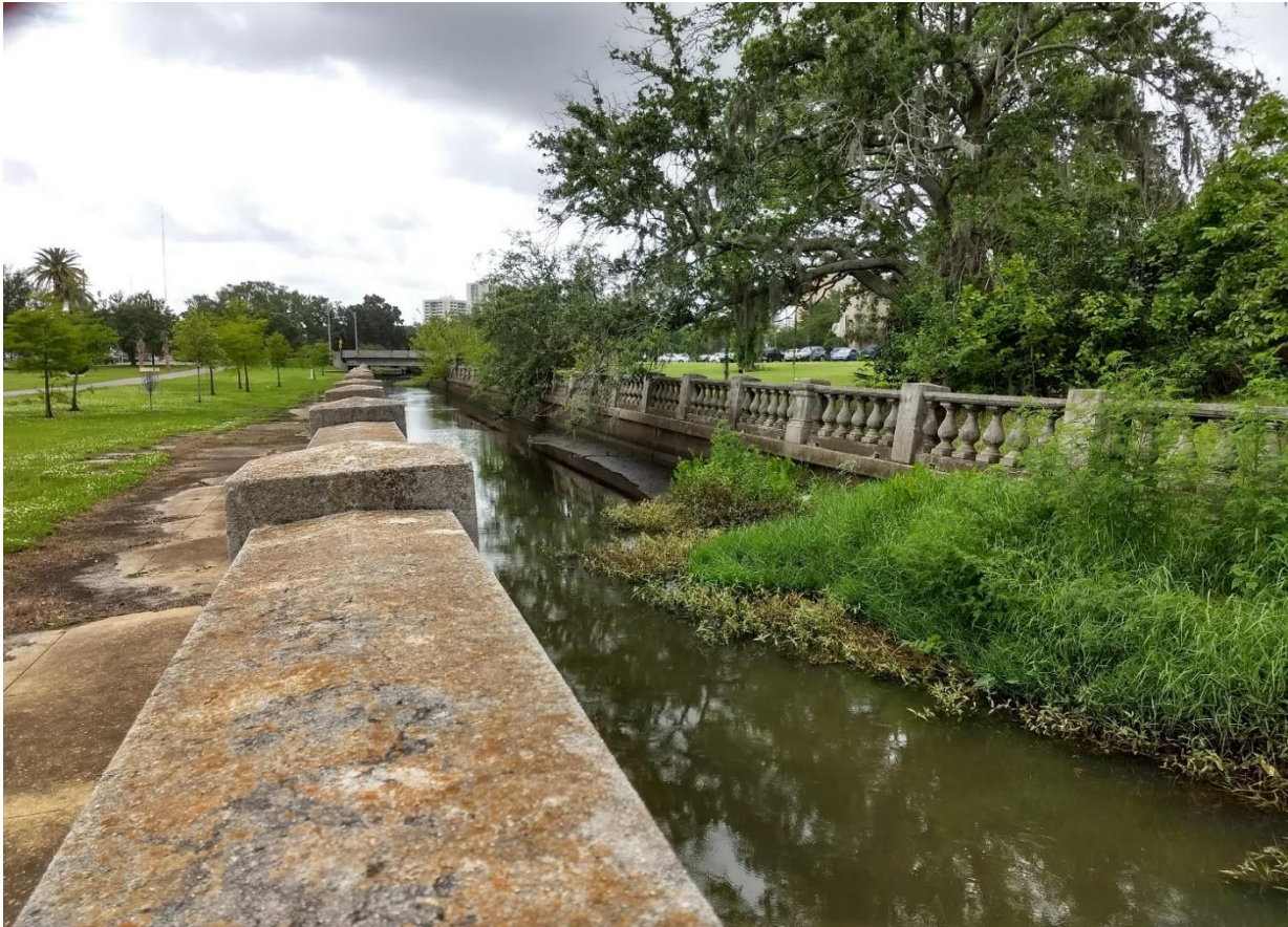
Figure CS2-1. Aging balustrades along Hogan's Creek in downtown Jacksonville.
