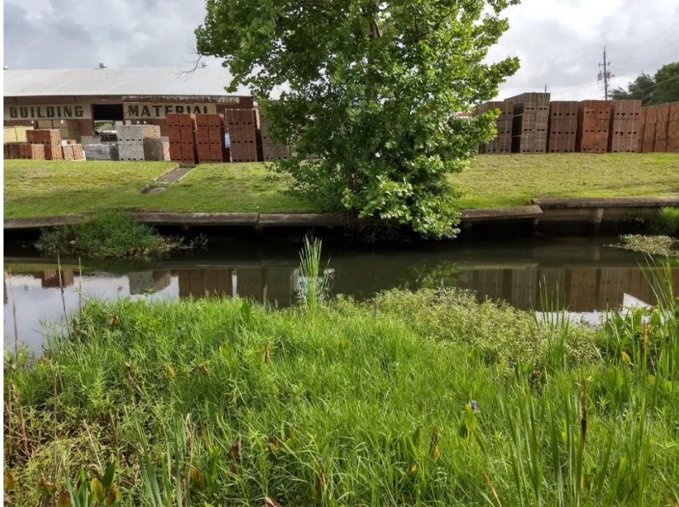
Figure CS1-7. Degrading bulkhead along a central segment of McCoy Creek. This area is also within the known soil contamination zone.
