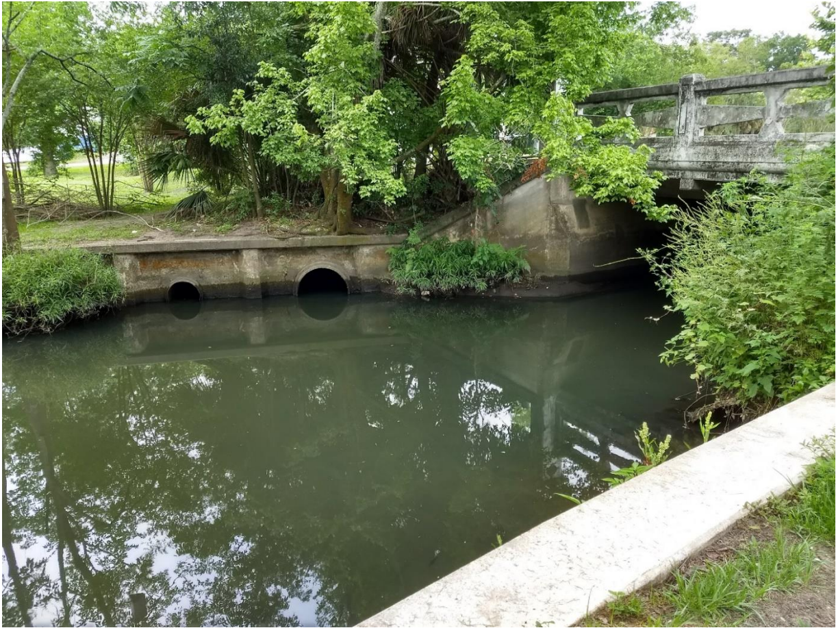
Figure CS1-1. Photo of McCoy Creek showing direct stormwater inflow and channel restricted by bridge.
