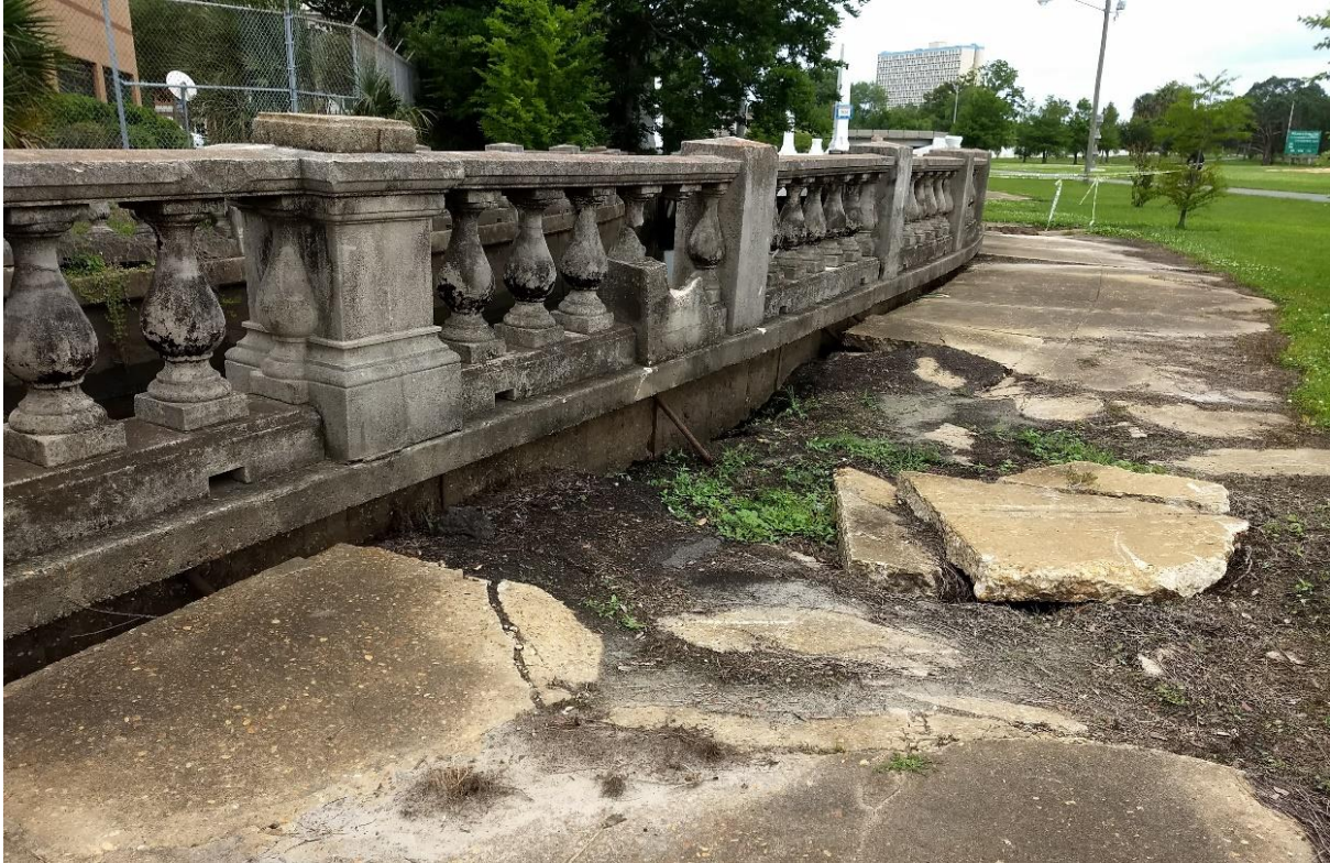
Figure CS2-7. Erosion has heavily damaged portions of historical balustrades along the creek.
