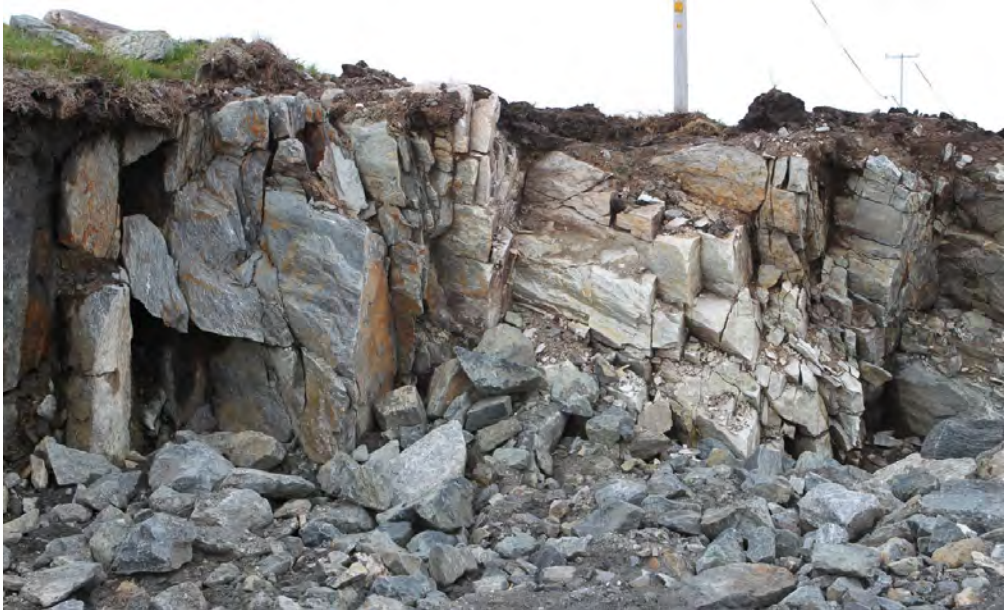
Figure 5.24 The bedrock in foundation 2.6 in the Mehuken II wind mill park consists of relatively competent amphibolite (Photo: Ragnar Hagen). The bedrock was investigated at depth through a 21,75 m long drill core that has been drilled towards the southwest with an inclination of 70 degrees from the horizontal (Göthfors 2010 and Appendix 2). The drill core consists of grey foliated augen gneiss. There are also some smaller segments of amphibolite. The augen gneiss is rich in mica minerals. The eyes are light in colour and often slightly extended in the foliation plane. The colour of the amphibolite varies from grey to greyish green to carbon black. The carbon black amphibolite is soft and crumbly. The dominant joint set is parallel to the foliation in the core. The core indicates a relatively fresh bedrock, but there are a few zones where the drill core is heavily fractured or totally crushed. There are not much secondary mineral filling in the fractures. Occurring fracture minerals are chlorite and calcite.
