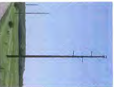
Transmission lines, such as those Great River Energy builds, deliver large or “bulk” amounts of electricity. After that, smaller distribution lines carry electricity to homes, farms and businesses. Pictured is a common structure for 69-kV and 115-kV transmission lines.
