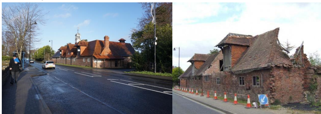
Sion Stables photo Marianne O’Kane Boal. Sion Stables before restoration. Photo copyright © NIFHA 2012
