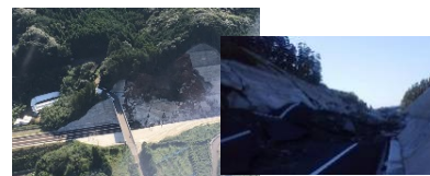
An example of road functions being affected by run-off of bridge superstructure or clogged road.
