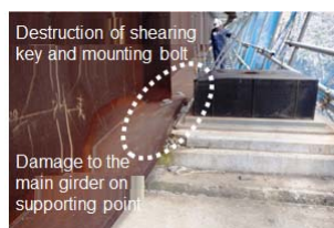
Fig. 1: Example of damage to the bridge bearing by the Kumamoto Earthquake
