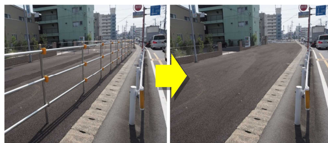
Fig. 2 Example of "Active and effective use of space" Removal of single pipes and use of road-widening site as provisional sidewalk space will greatly improve user-friendliness.
