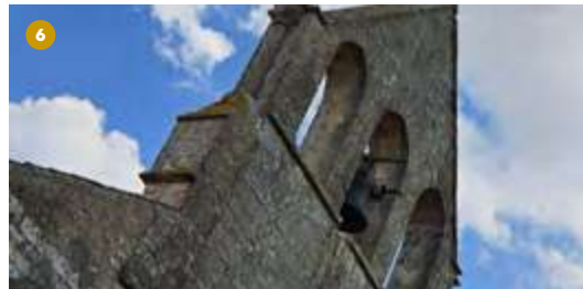
6 Saint-Martin-de-Bernegoue Saint-Martin church, original by its beautiful belfry at the top of the choir's entry, with three arcades for the bells.
