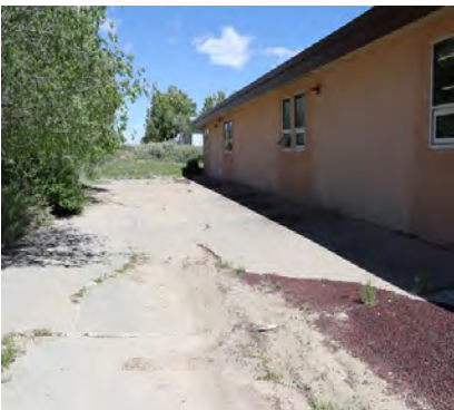
Cimarron School Campus settlement and cracking of drainage diversion dam behind High School building.
