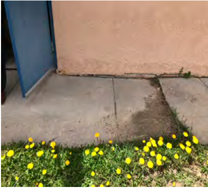
School building damage caused by drainage problems.
