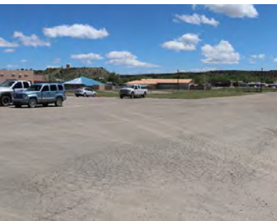
Cimarron High School parking lot asphalt cracking.
