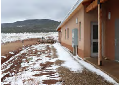
Moreno Valley High School site erosion from roof drainage on North Side of building.
