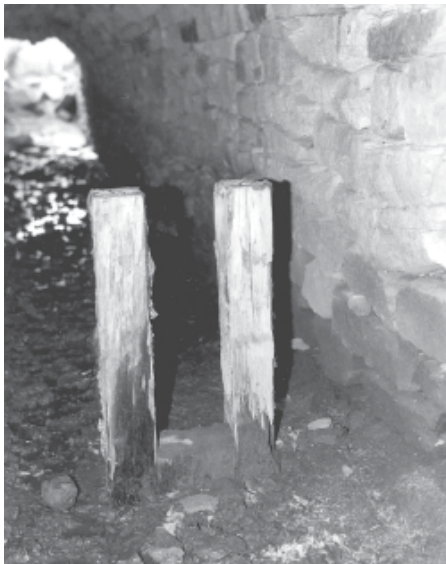
PLATE 6. Typical spear rod support, Jeffrey's east end. The sheaves supported a pulley wheel upon which the round bars rested (1986).
