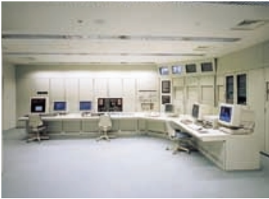
Fire Monitoring Panels in Control Center
