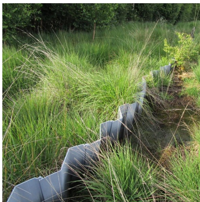
Drain blocking at Wem Moss (15 th June)
