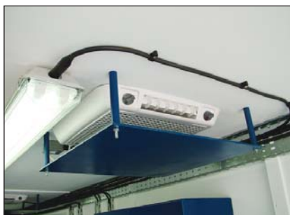
Roof mounted air conditioners
