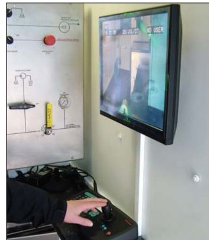
Flat screen monitor and CCTV controls
