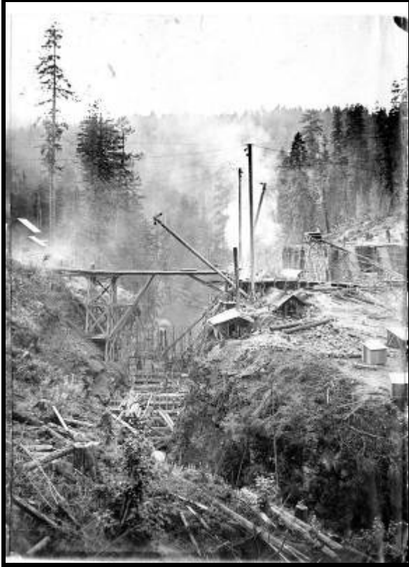
Figure 35. Early stages of construction of the Elwha Dam spillway and powerhouse, looking upstream, ca. 1910-11. Photograph by Critchfield. Courtesy of Clallam County Historical Society, ONP ref. no. 2010.200.145. [2010200145.JPG]
