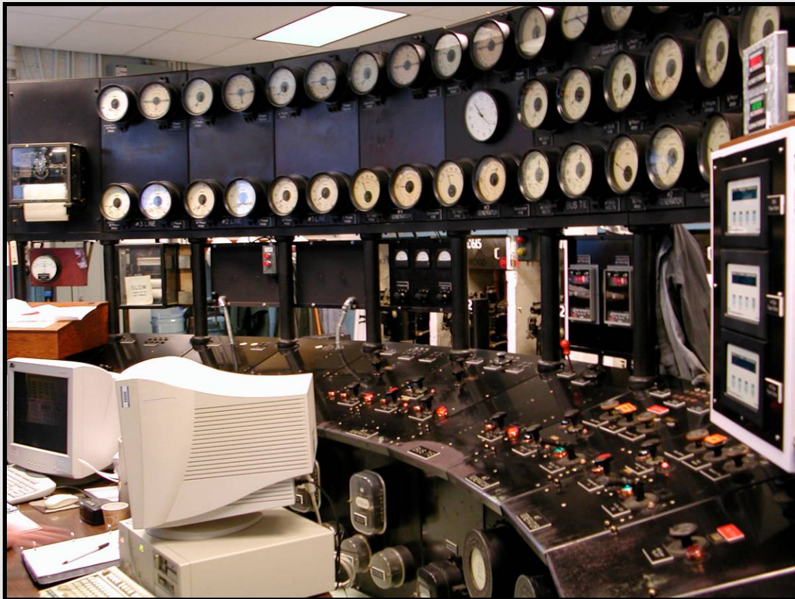
Figure 109. Control panels at the Elwha Dam, 2005. Photograph by Betsy Carlson. Courtesy of Olympic National Park. [Elwha Dam Control Panels.jpg]
