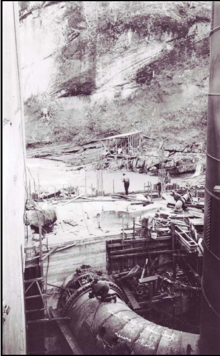
Figure 61. Construction of intake at Glines Canyon Dam, ca. 1926–1927. Courtesy of Olympic National Park. [HAER_OLYM437_SlemmonsElwha1.TIF]
