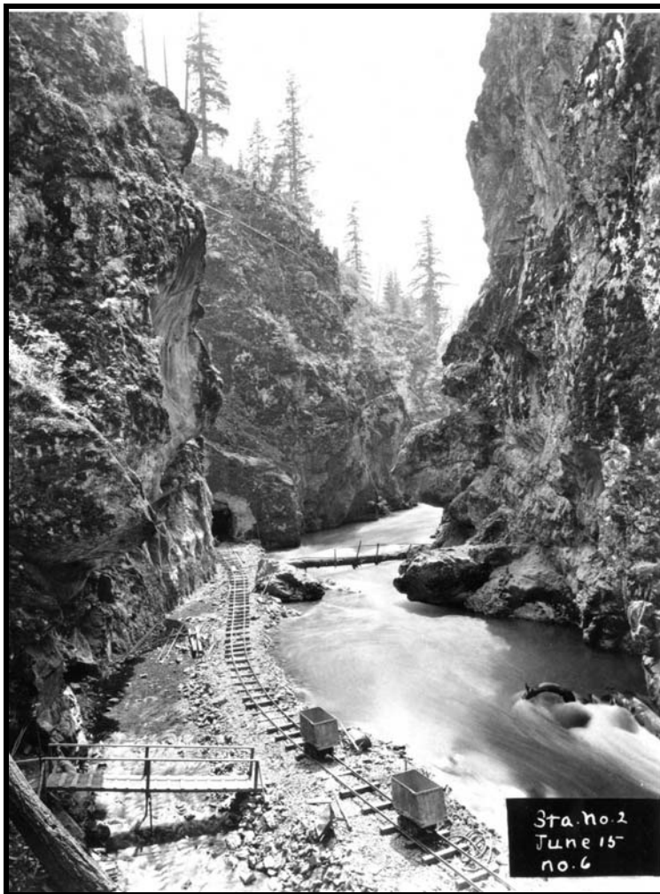
Figure 62. Diversion tunnel at Glines Canyon Dam, June 15, [1927]. The river was diverted through this tunnel while dam construction was underway. Courtesy of Clallam County Historical Society, ONP ref. no. 2010.200.135. [2010200135.JPG]
