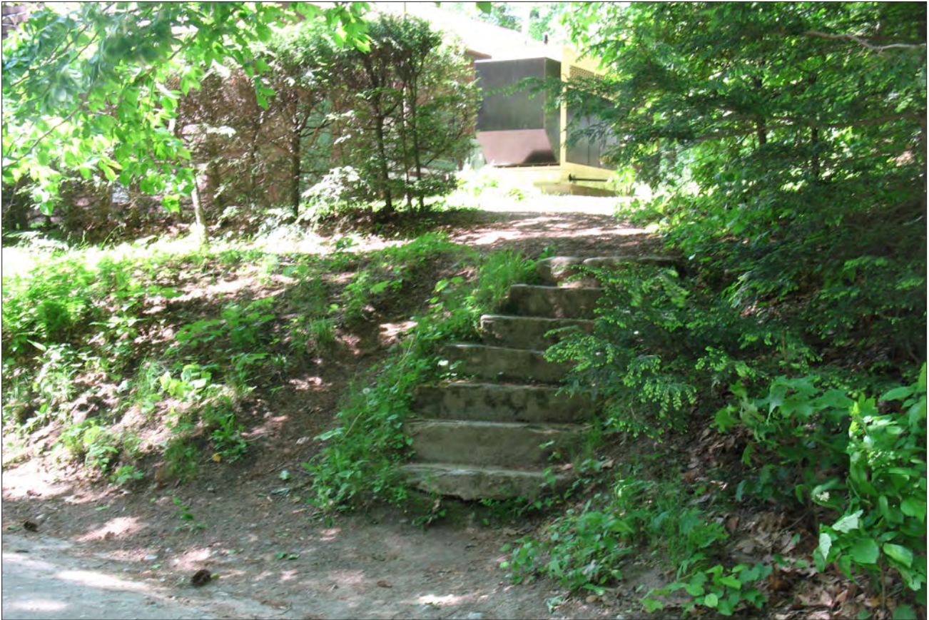
Figure 62. View northwest of the mortared fieldstone steps from Saint Gaudens Road to the southeast corner of the property, behind the visitor center (OCLP, 2009).
