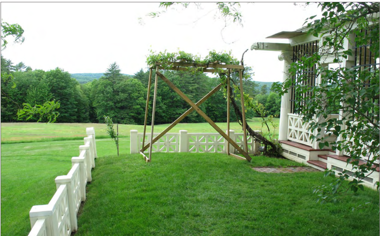
Figure 19. View west of the terrace balustrade, newly planted poplar, grape vine, lilac, brick walk, and piazza at the southwest corner of the house. The grape vine rests on a temporary structure while repairs are made to the piazza roof. The west meadow is visible in the background with Juniper Hill in Vermont partially visible in the distance (OCLP, 2009).
