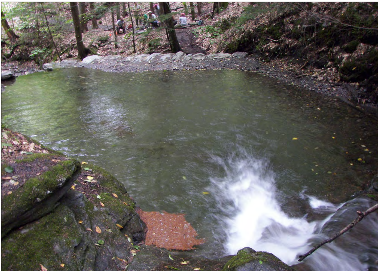
Figure 57. View east of the swimming hole and dam along Blow-Me-Up Brook in the ravine below Aspet after repairs (SAGA, 2008).
