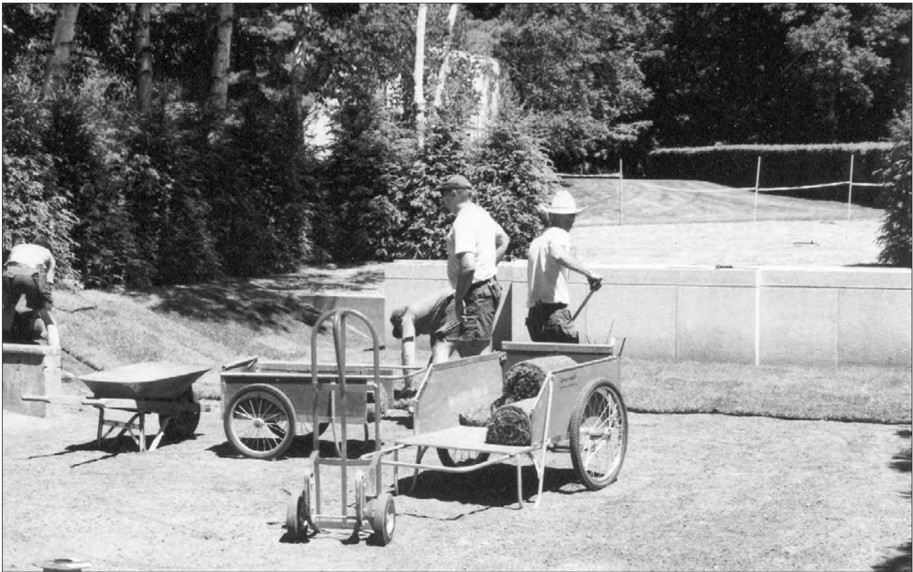
Figure 3. Laying sod at the newly constructed Shaw Memorial base. Hedges east of the statue base were removed to provide access to the area and the area was regraded (SAGA, 1997).
