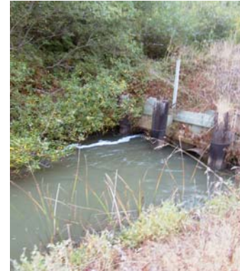
Leaky gate on Fish Hatchery Creek
