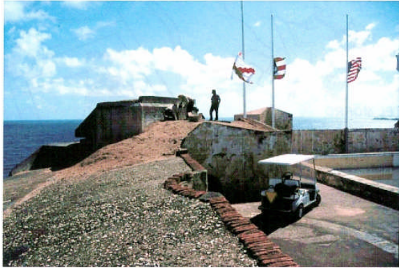
Figure 6: Roofs of the rooms (casemates) on the north edge of the Plaza de Armas in El Morro were filled with dirt to provide protection against shell bombardments from enemy ships approaching from the Atlantic Ocean. Several pieces of wood with apparent termite damage were found on top of the roofs, and activity of C. havilandi (MORO2) and Heterotermes sp. (MORO3) were detected by stake survey.
