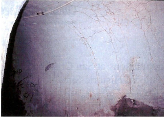
Figure 1: Old and hardened foraging tubes of Heterotermes sp. were found on the walls of underground tunnels in San Cristóbal, and are indicative of a long presence of this endemic species within the fortress.
