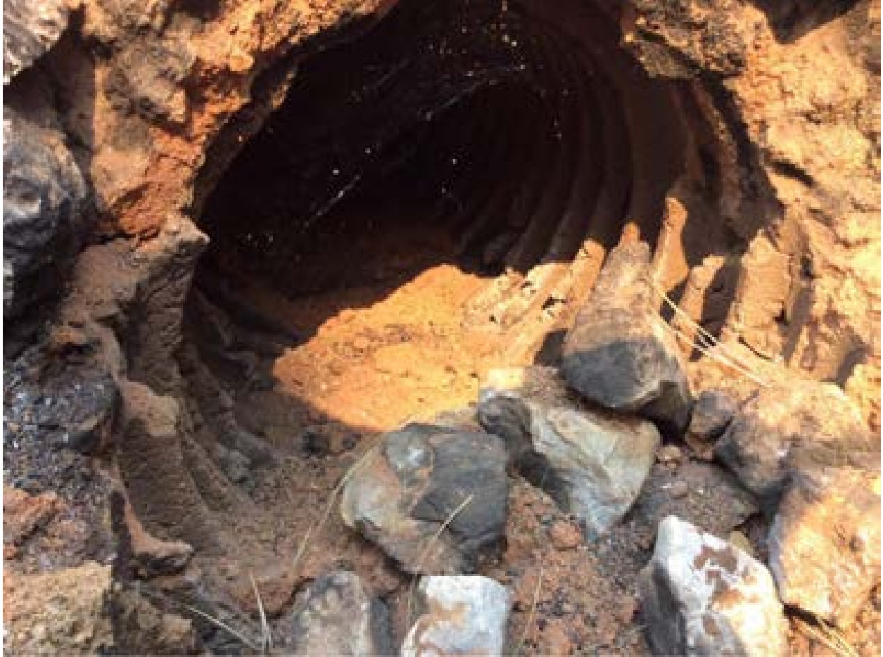
Burned plastic culvert on Sacramento River Rail Trail
