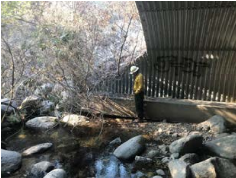
Erosion under concrete footer at Boulder Creek road crossing.
