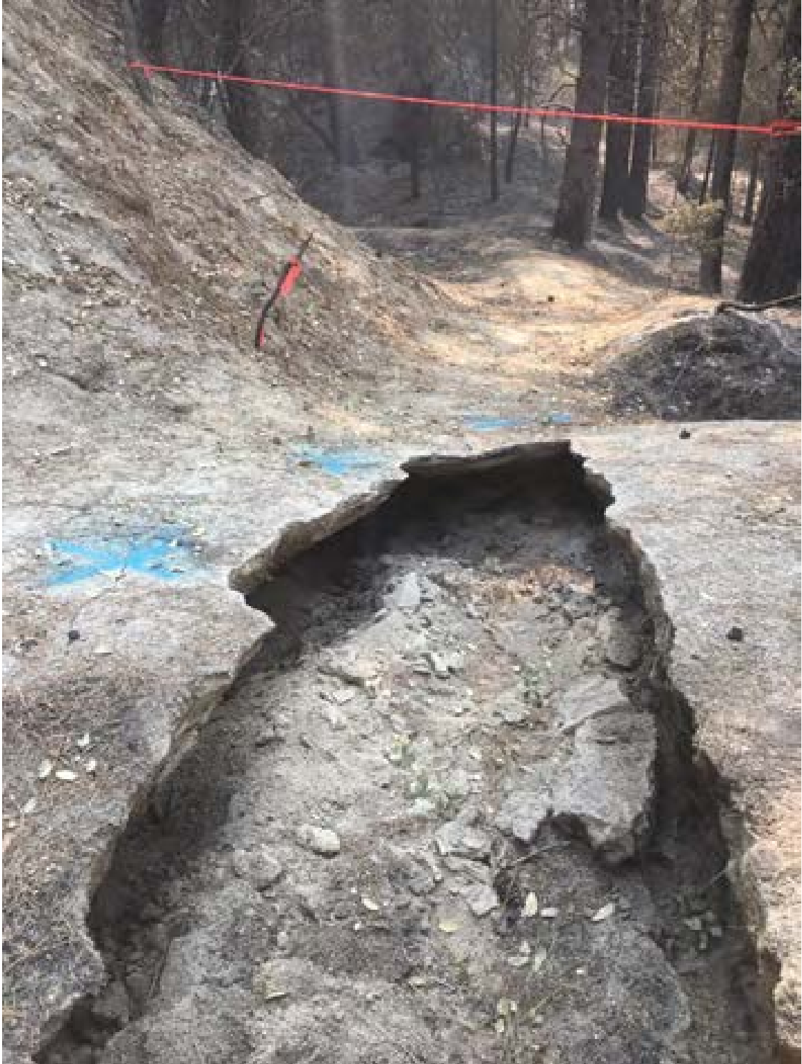
Collapsed Trail Tread – Whiskeytown Falls Trail
