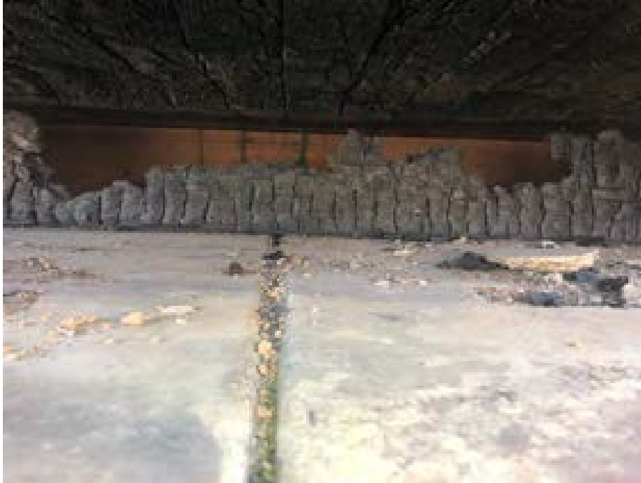
Crystal Creek Storage Tank, burned floorboards, joists, and concrete pad, 8/15/18.
