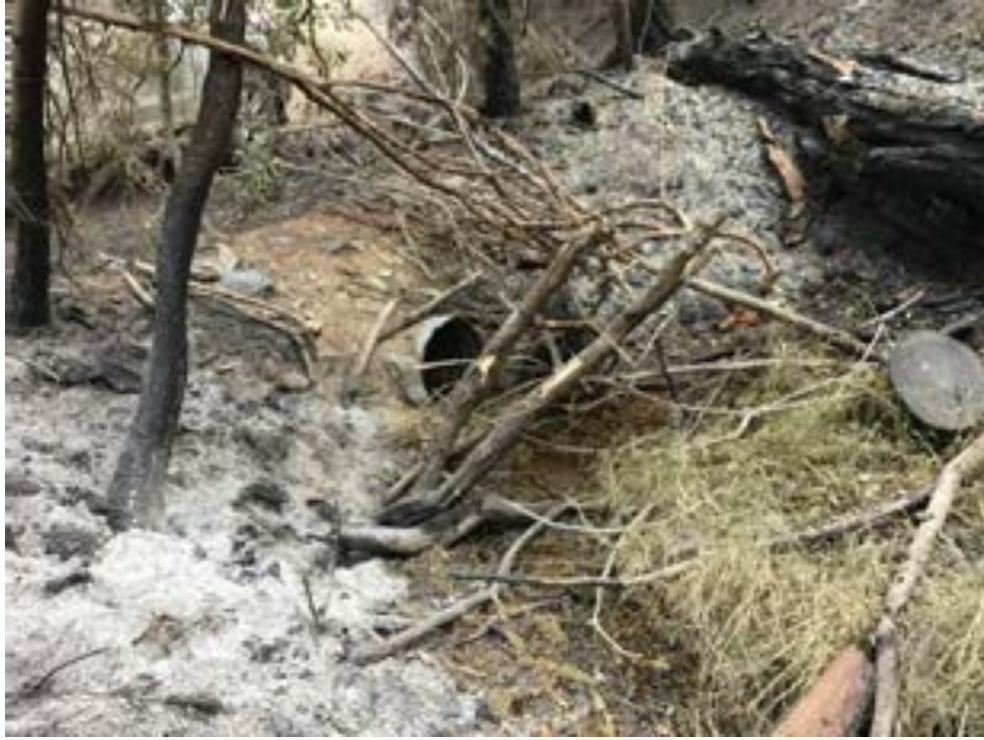
Fire-related debris clogging culvert inlet and need of cleaning prior to storm events.
