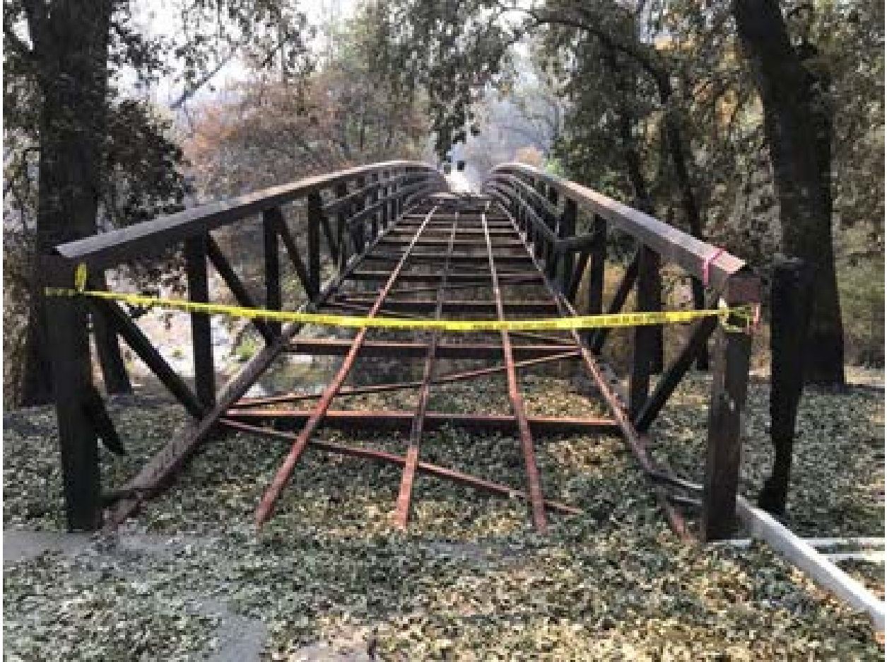
Burned Bridge between Mill Creek Trail and Tower House parking
