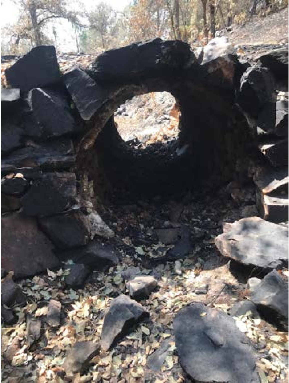
Burned Culvert on Mule Ridge Trail
